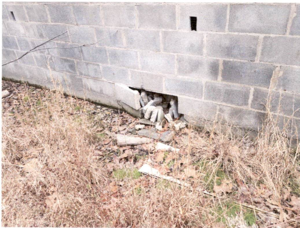
Damaged Right Foundation Wall
