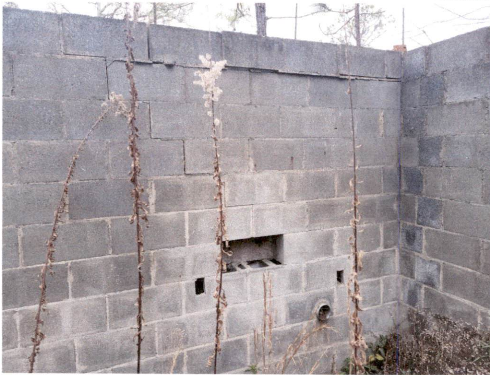
Damaged Back Foundation Wall
