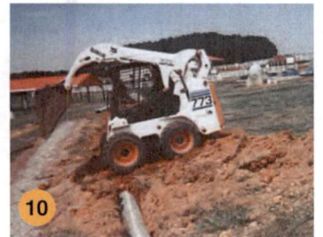
10 Narrow trenches allow for faster, less cumbersome of equipment about the site during the final cover phase, and this saves equipment time on the job.
