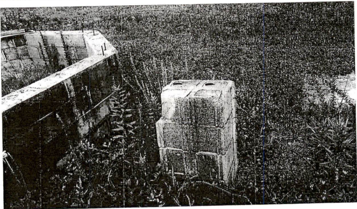
Item 2b) Examples of damaged piers to be repaired
