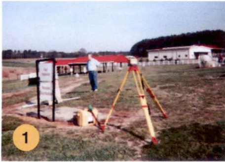
1 NC State University layout of CPP No-Rock Septic at the Ed Booth field Learning Lab.
