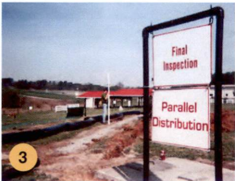
3 Laser Level check of trench depth grade and bag encased protected pipe moved onto trench site. The plastic bags protect the filter wrap from extended storage UV deterioration and natural handling abuses.
