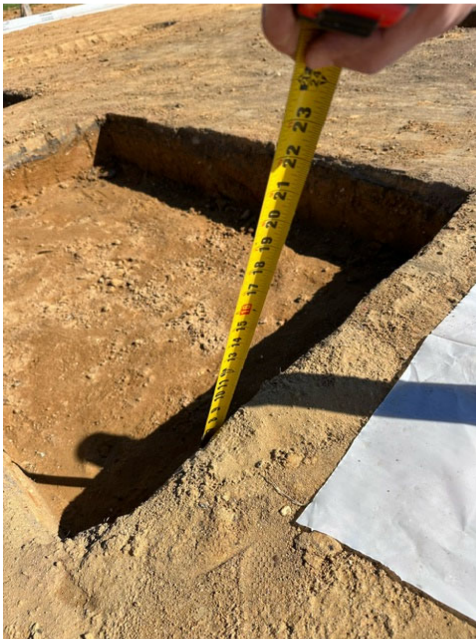
Figure 4.0 Depth of footing (12")
