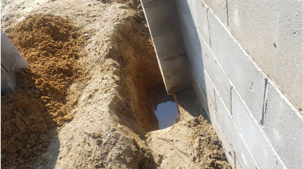
Examples and locations of piers with inadequate footing projection
