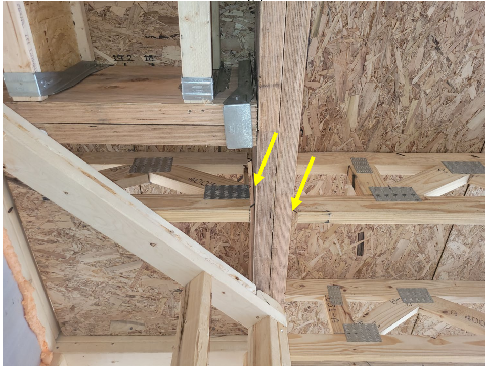
Furr out LVL w/ OSB to fill gap between truss and LVL.
