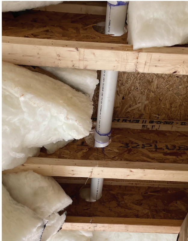
Photo 1: existing holes in webbing of TJI-joist
