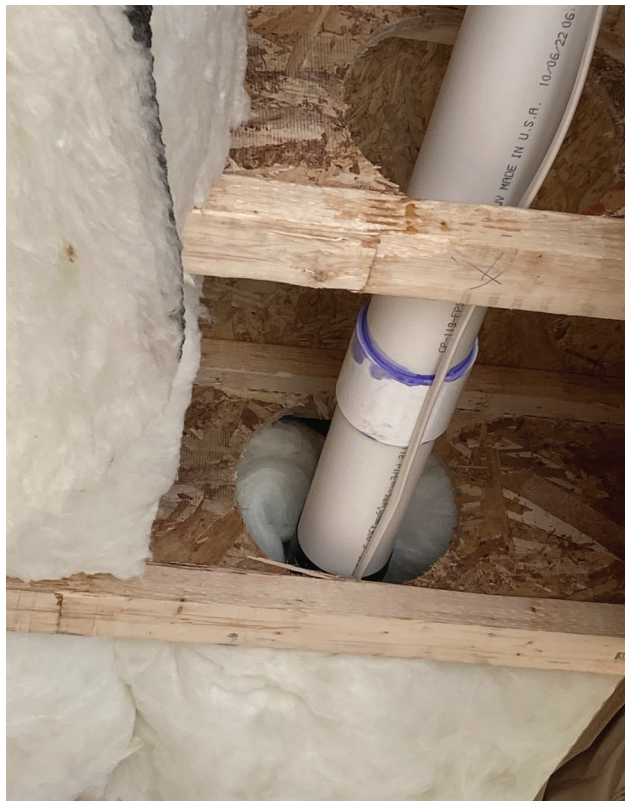
Photo 2: existing holes in webbing of TJI-joist
