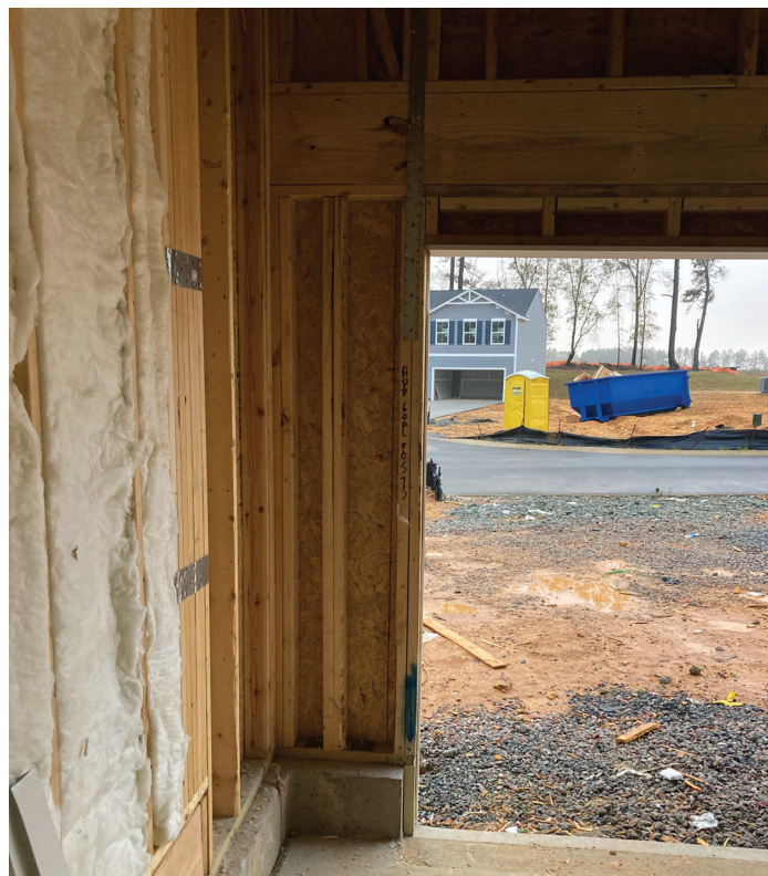
Photo 2: framing overhang observed at garage portal wall
