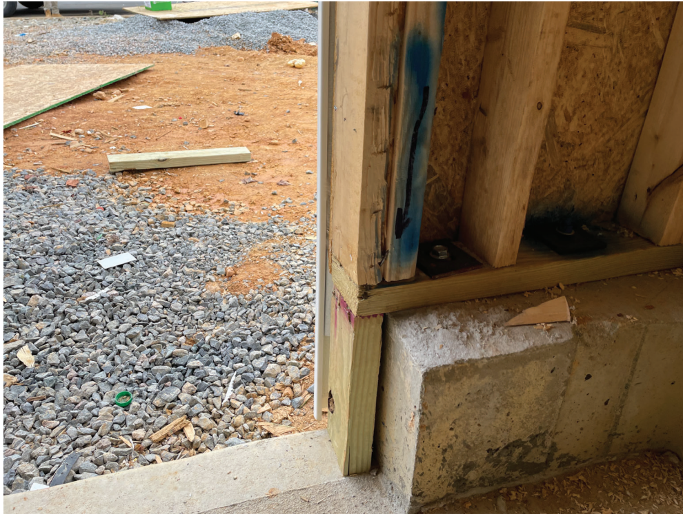
Photo 1: framing overhang observed at garage portal wall
