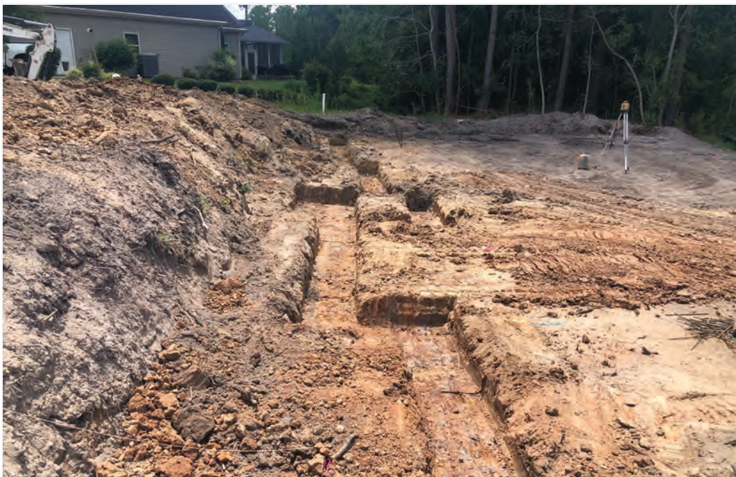
Site conditions observed, heavy organics observed, prior to contractor removing
