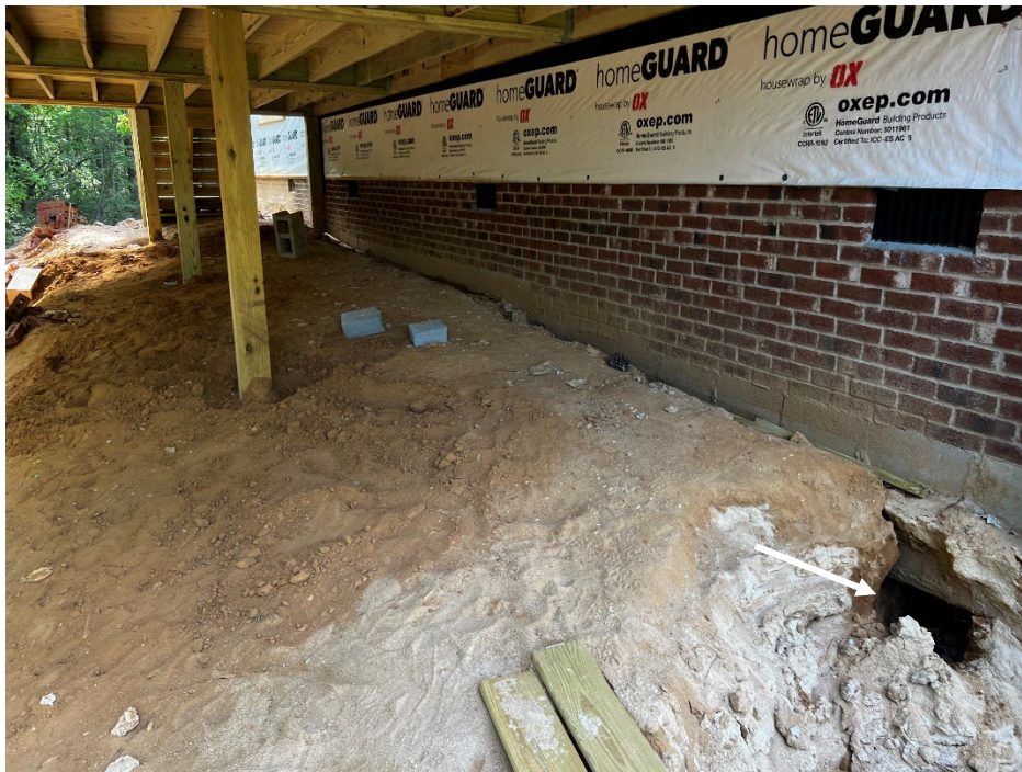
Picture 4: Footing Undermine
