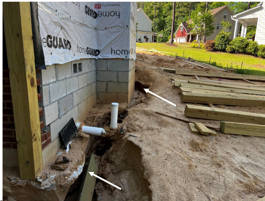
Picture 2: Foundation Support Eroded, Trench/Slope Along Foundation
