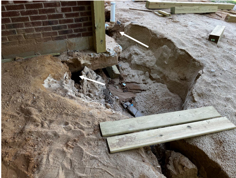
Picture 1: Foundation Support Eroded, Trench/Slope Along Foundation
