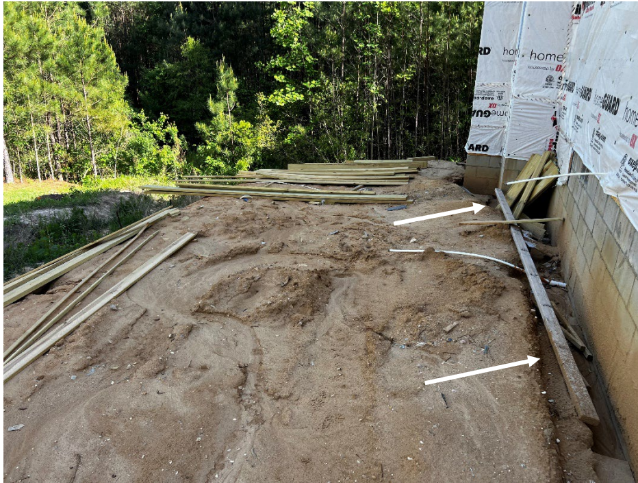
Picture 3: Negative Slope/Trench
