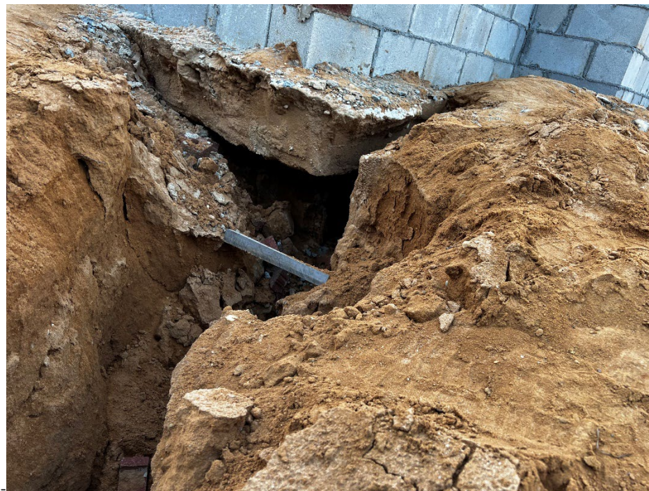
Picture 2: Foundation Support Eroded
