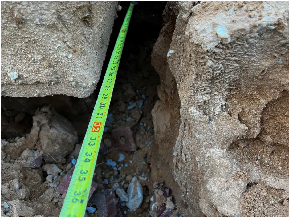
Picture 5: Depth of Footing Undermine
