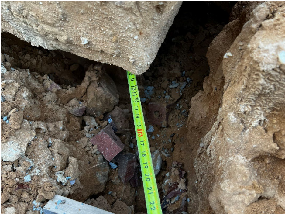
Picture 6: Depth of Footing Undermine
