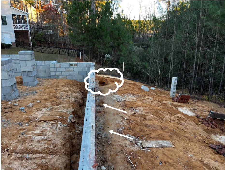
Picture 3: Location of Footing Undermine, Negative Slope/Trench
