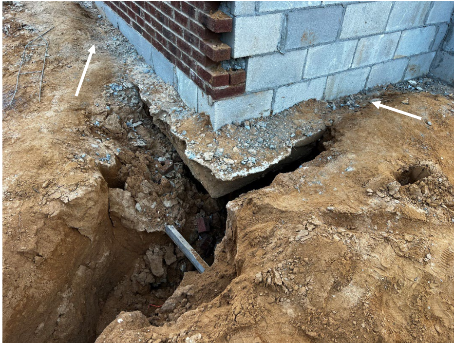
Picture 1: Foundation Support Eroded, Trench/Slope Along Foundation
