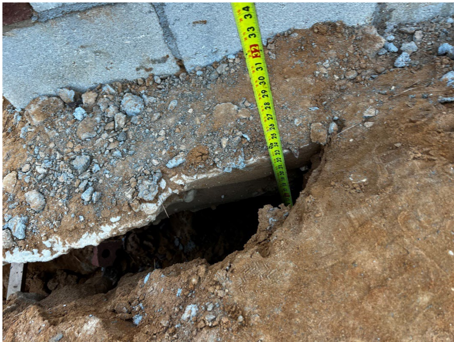
Picture 4: Depth of Footing Undermine
