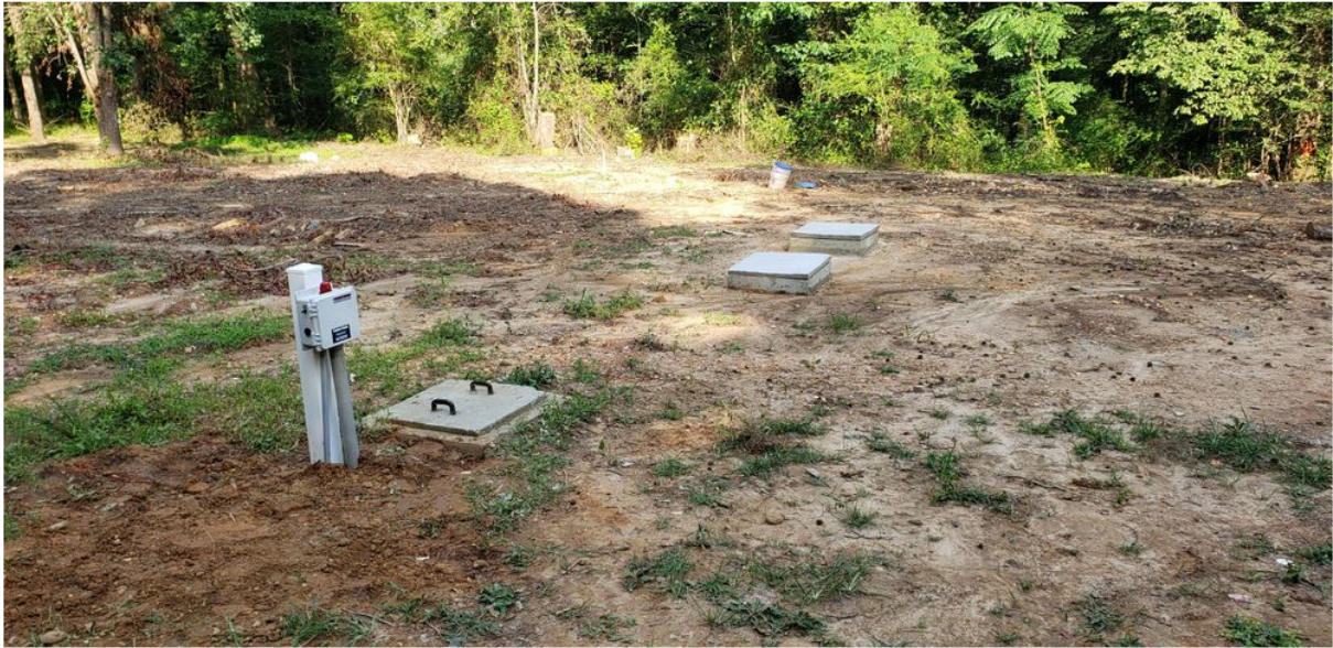
View of Control Panel Installed
