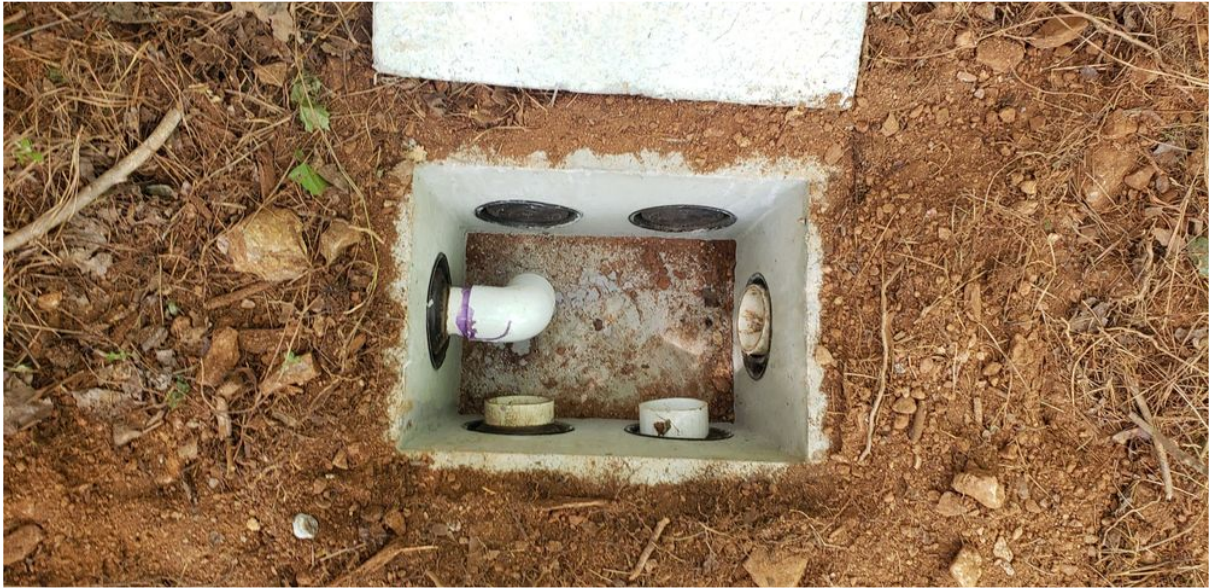
View of Inside of Distribution Box
