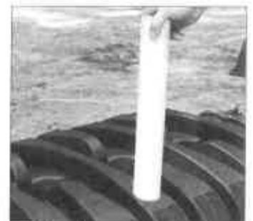
Chamber inspection port.
