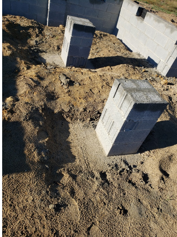
Example of Piers outside Center Third of Footings
