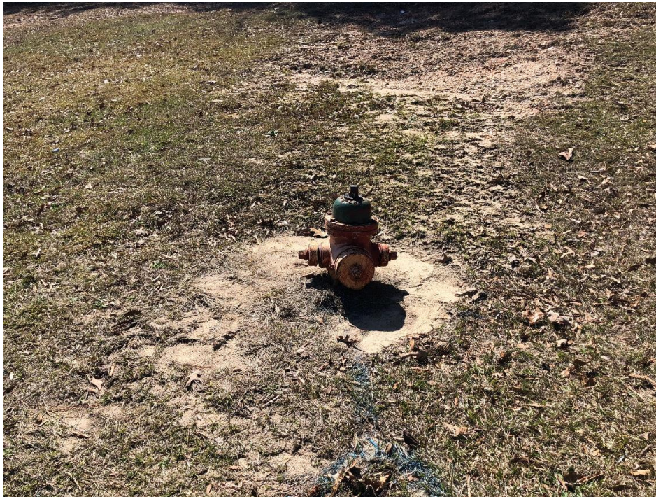
Photograph 2. Fire Hydrant (Pressure Hydrant) located to the west of Lillington Shawtown Elementary.
