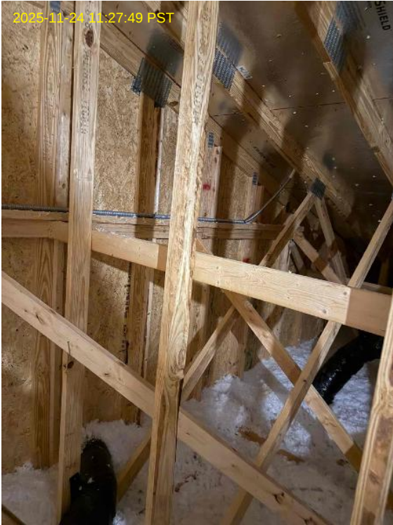
Internal Installers Loc: 35.6032, -78.8168
