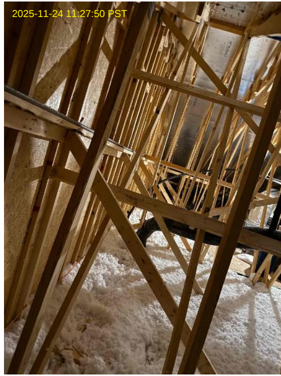
Internal Installers Loc: 35.6033, -78.8168
