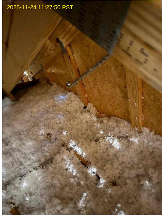
Internal Installers Loc: 35.6032, -78.8169
