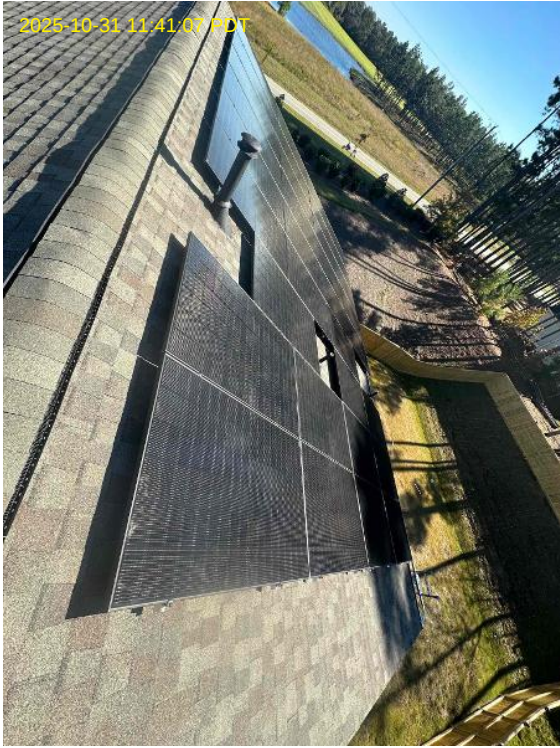
Roof Photos / Array 1 / Complete Array with all modules visible + Rail trimmed
