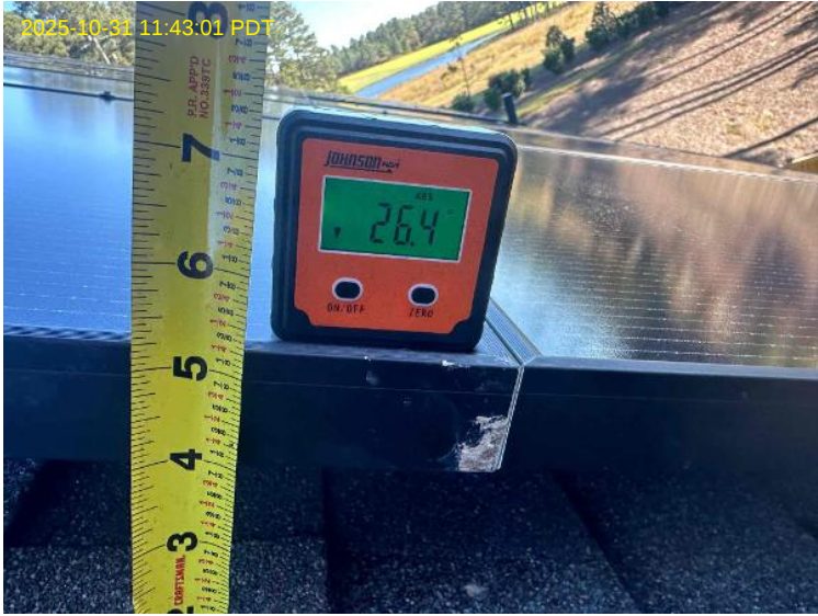
Roof Photos / Array 1 / Tilt - measured on array
