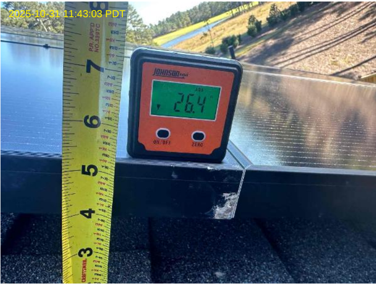
Roof Photos / Array 1 / Tilt - measured on array
