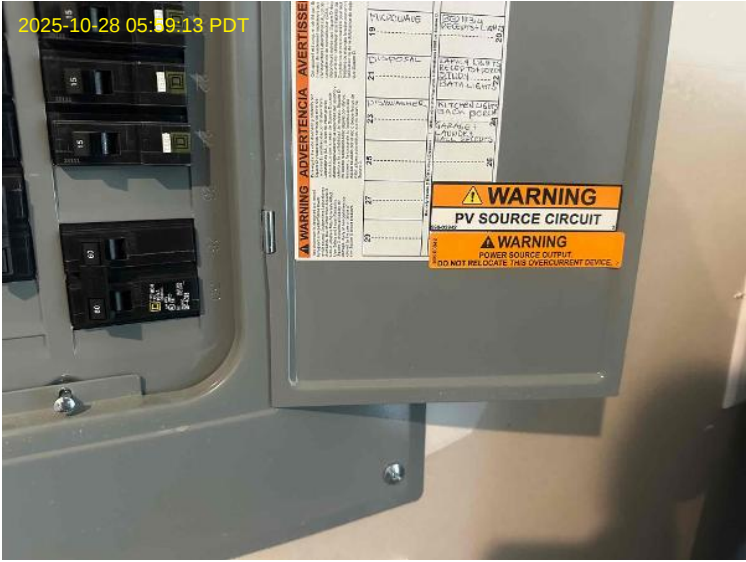
Electrical photos / Point of Interconnection - Close up
