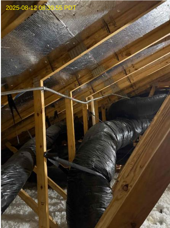
Internal Installers Loc: 35.5016, -78.8054
