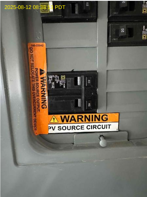
Electrical photos / Point of Interconnection - Close up
