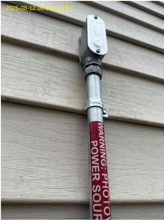
Internal Installers Loc: 35.5014, -78.8054
