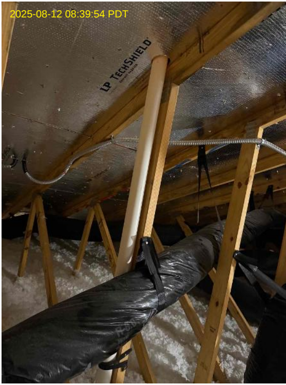
Internal Installers Loc: 35.5016, -78.8055
