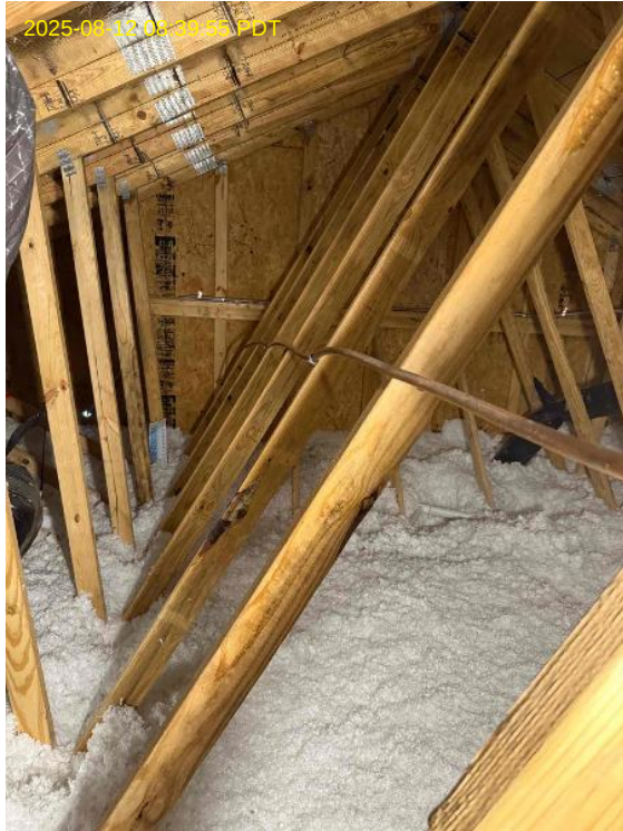
Internal Installers Loc: 35.5017, -78.8052
