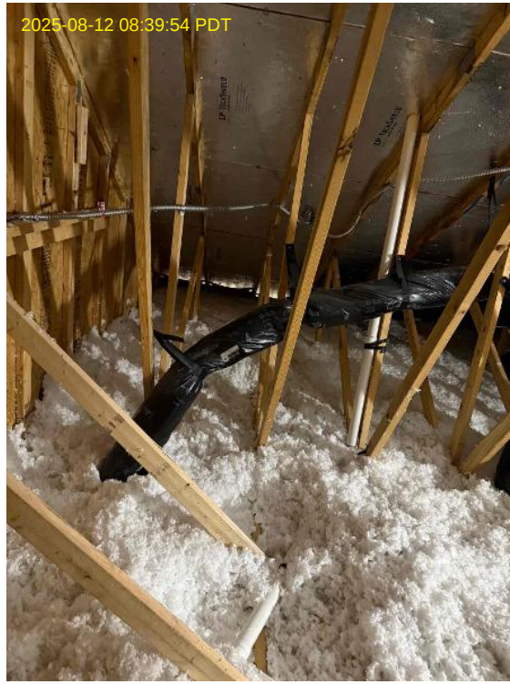
Internal Installers Loc: 35.5017, -78.8056
