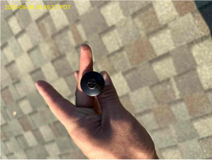
Roof Photos / Photo: Mid Clamp
