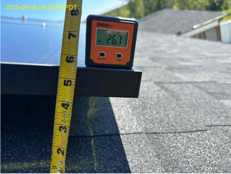
Roof Photos / Array 1 / Tilt - measured on array
