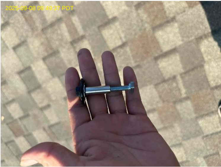
Roof Photos / Photo: Mid Clamp
