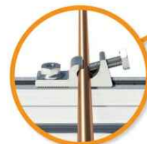
Grounding Lug A single Grounding Lug connects an entire row of PV modules to the grounding conductor.
