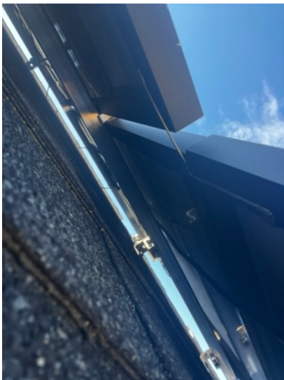
Detailed picture of ENTIRE GROUND WIRE PATH ON RACKING
