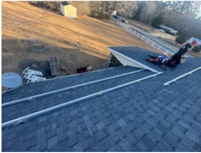
Detailed picture of complete racking installed
