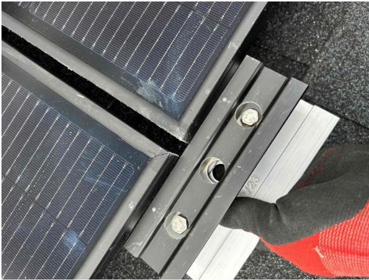
Rooftop Installation / Appropriate Racking Markings
