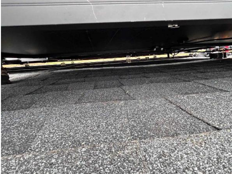
Rooftop Installation / Wire management Under the Array (1 photo per row of modules per array)
