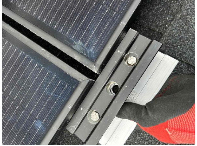
Project Completion Photos / Appropriate Racking Markings
