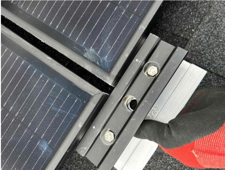
Rooftop Installation / Appropriate Racking Markings
