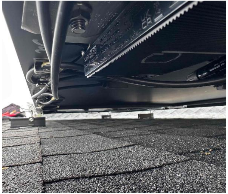
Rooftop Installation / Wire management Under the Array (1 photo per row of modules per array)
