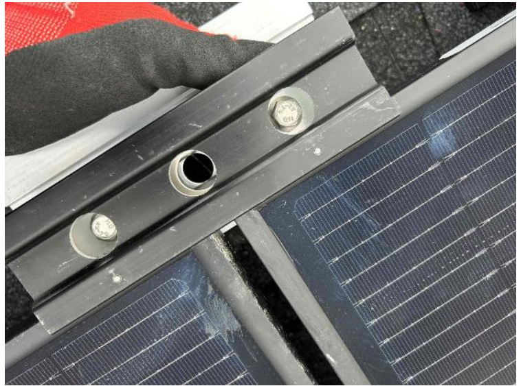
Rooftop Installation / Appropriate Racking Markings
