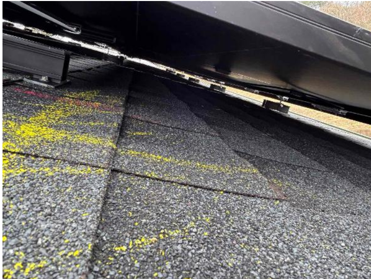
Rooftop Installation / Wire management Under the Array (1 photo per row of modules per array)
