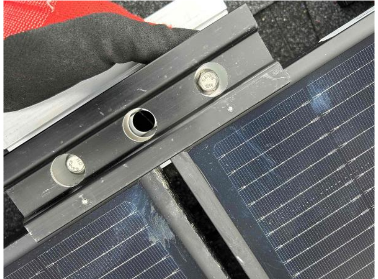
Rooftop Installation / Appropriate Racking Markings
