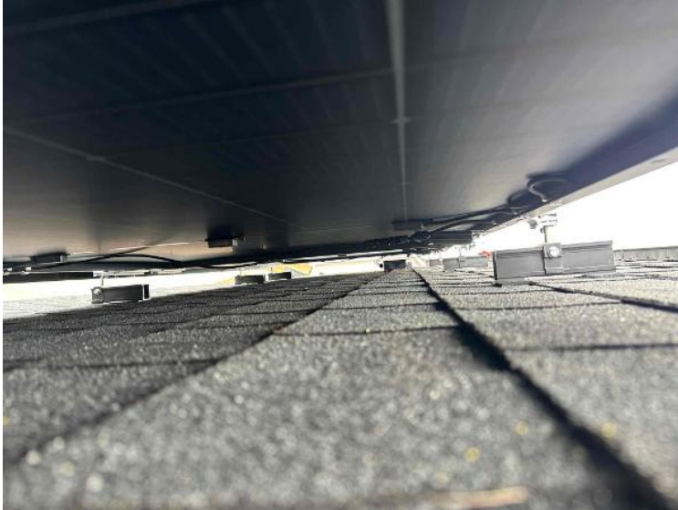
Rooftop Installation / Wire management Under the Array (1 photo per row of modules per array)
