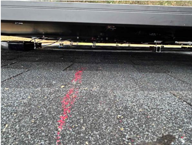
Rooftop Installation / Wire management Under the Array (1 photo per row of modules per array)
