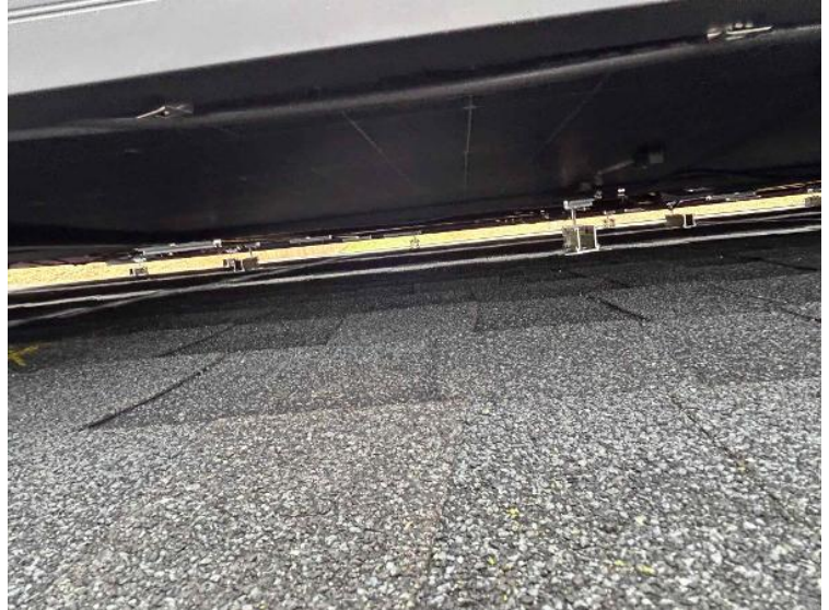
Rooftop Installation / Wire management Under the Array (1 photo per row of modules per array)
