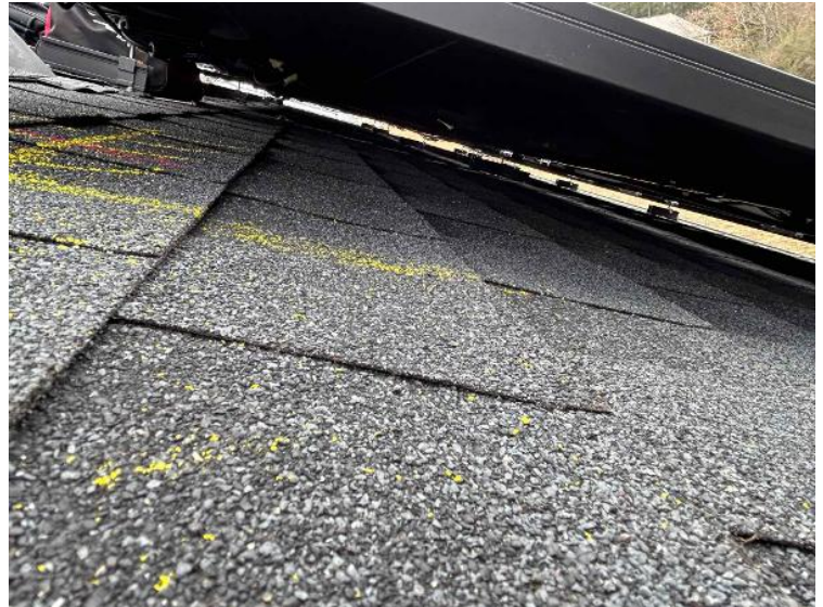
Rooftop Installation / Wire management Under the Array (1 photo per row of modules per array)
