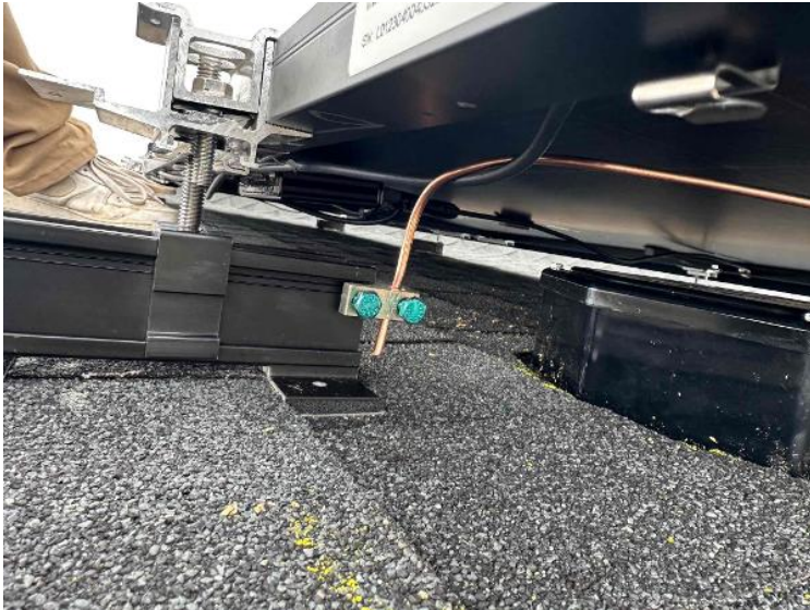
Rooftop Installation / Wire management Under the Array (1 photo per row of modules per array)
