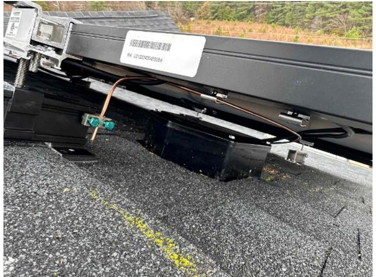
Rooftop Installation / Wire management Under the Array (1 photo per row of modules per array)
