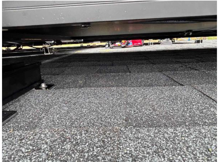
Rooftop Installation / Wire management Under the Array (1 photo per row of modules per array)
