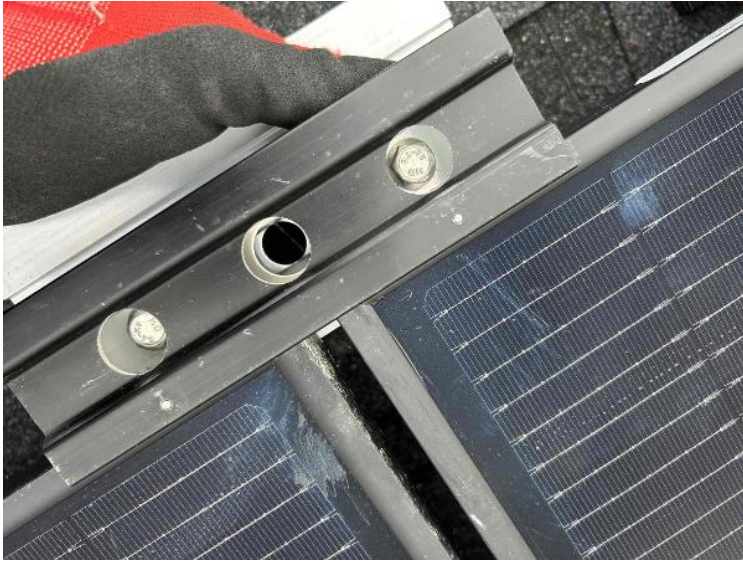
Project Completion Photos / Appropriate Racking Markings
