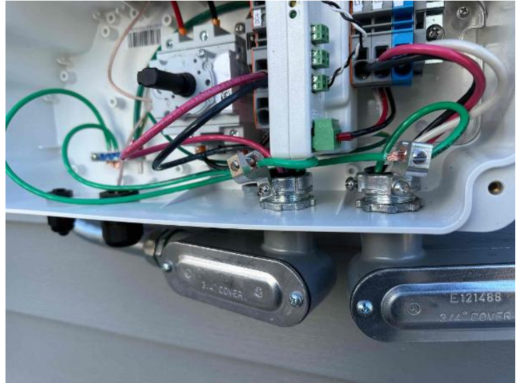
Electrical Installation / Inverter/Combiner Installed & Wired
