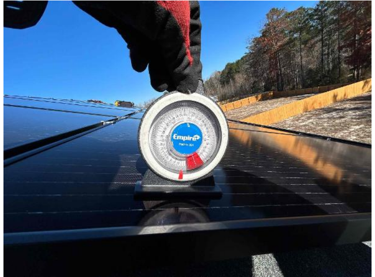
Project Completion Photos / Tilt photo: array 1
