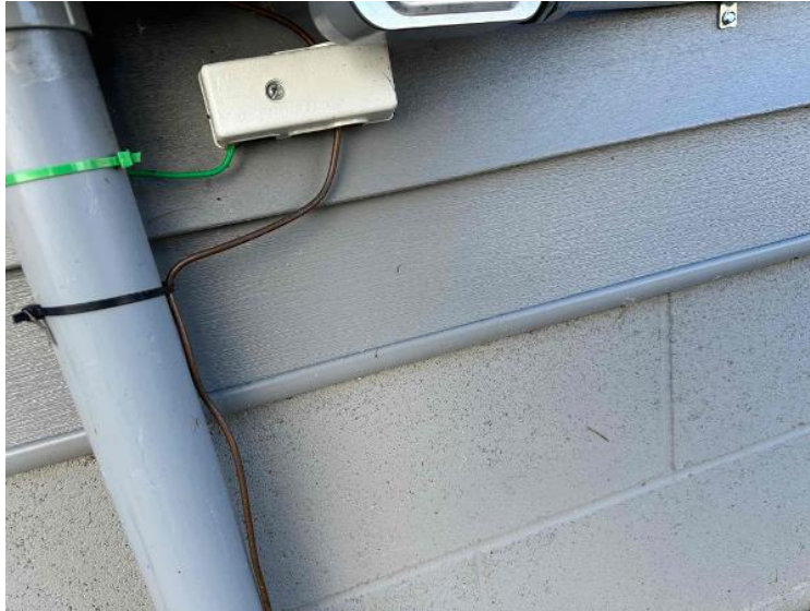
Electrical Installation / The Main Service Panel's GEC
