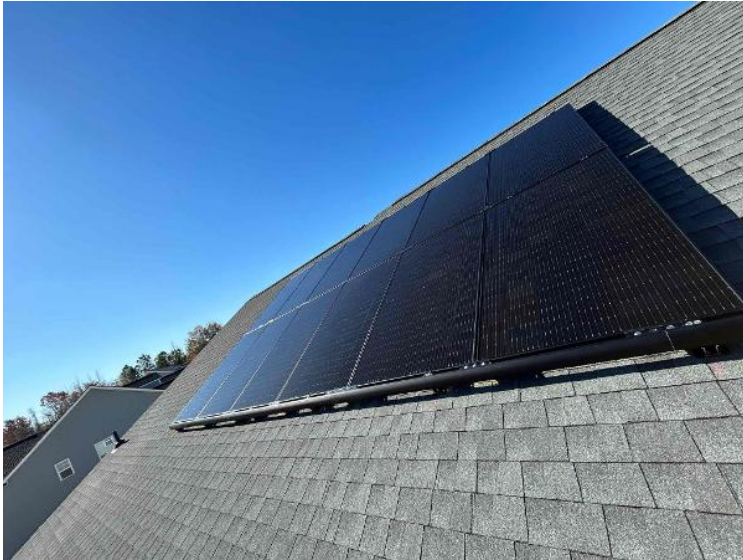
Project Completion Photos / Photo of array 1
