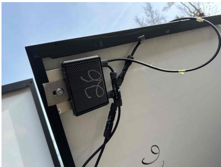
Crew Lead Review + Quality Assurance / Screenshot of Missing Adders
