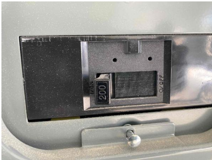
Electrical Installation / Close Up Photo of Panel Label + Main Breaker Rating on The Breaker
