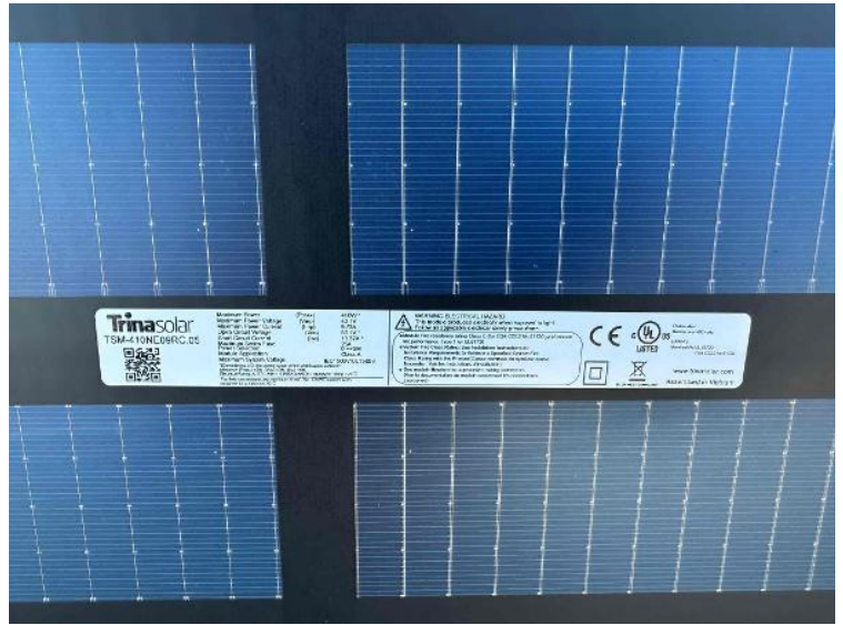
Rooftop Installation / Module Label
