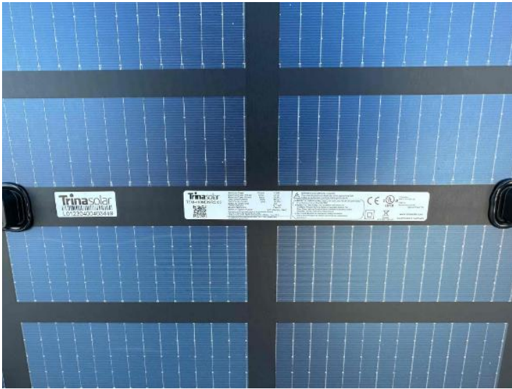
Rooftop Installation / Module Label
