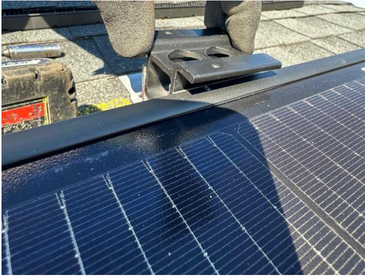
Rooftop Installation / Appropriate Racking Markings
