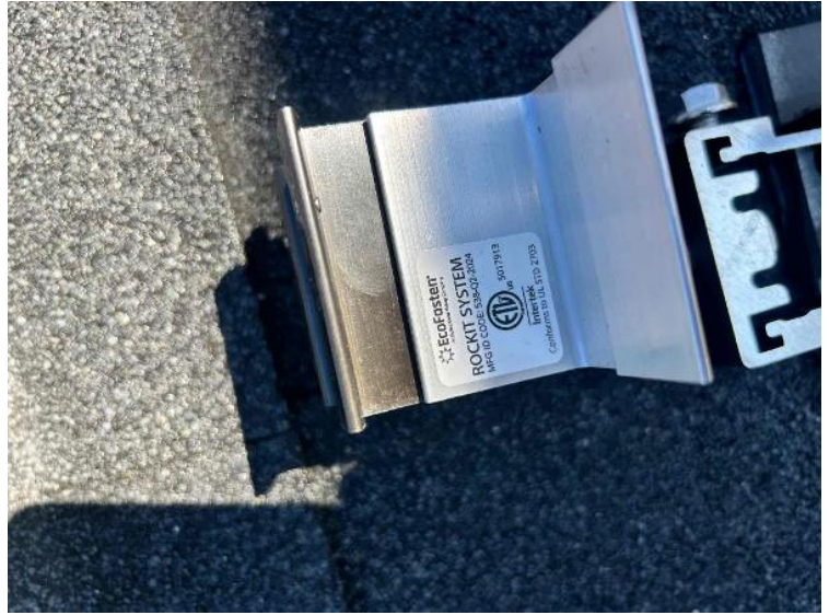
Rooftop Installation / Appropriate Racking Markings
