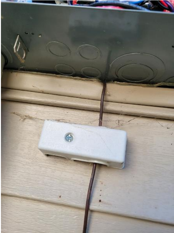
Electrical Installation / The Main Service Panel's GEC
