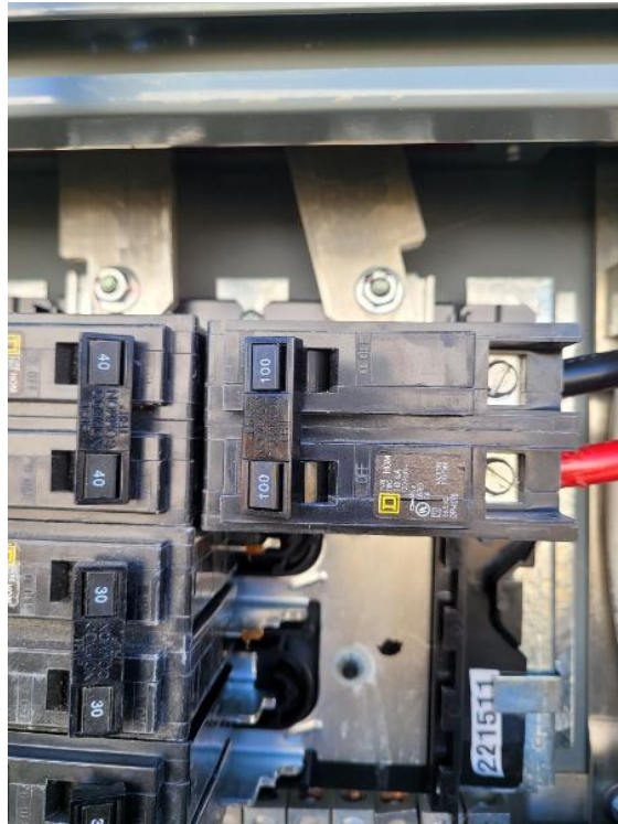
Electrical Installation / Close Up Photo of Panel Label + Main Breaker Rating on The Breaker
