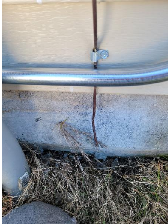
Electrical Installation / The Main Service Panel's GEC
