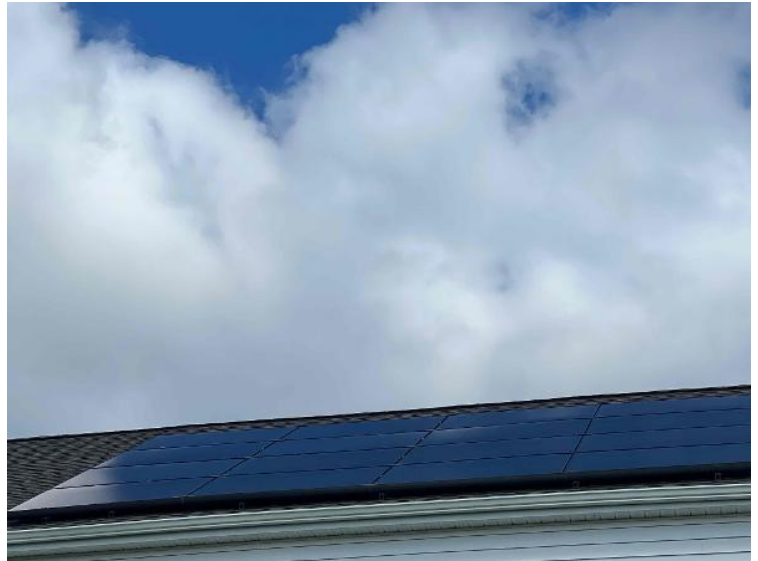
Project Completion Photos / Complete Array Photos (all modules MUST be visible in each array)
