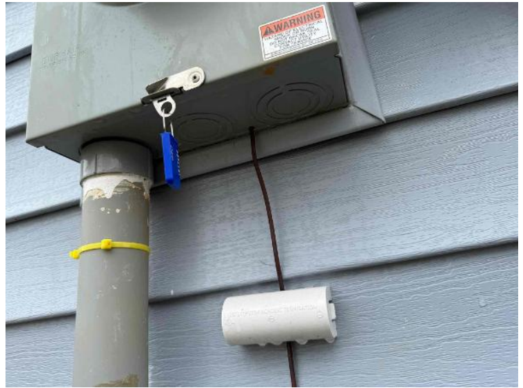
Electrical Installation / The Main Service Panel's GEC
