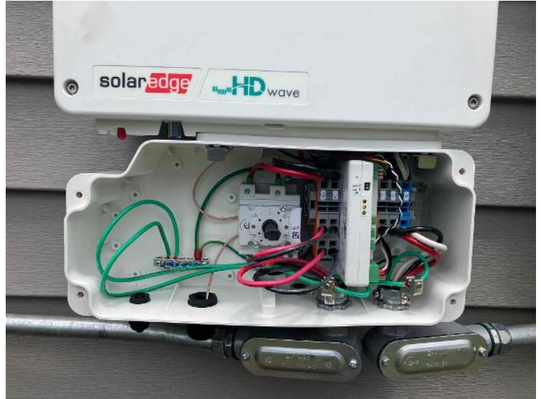
Electrical Installation / Point of Interconnection
