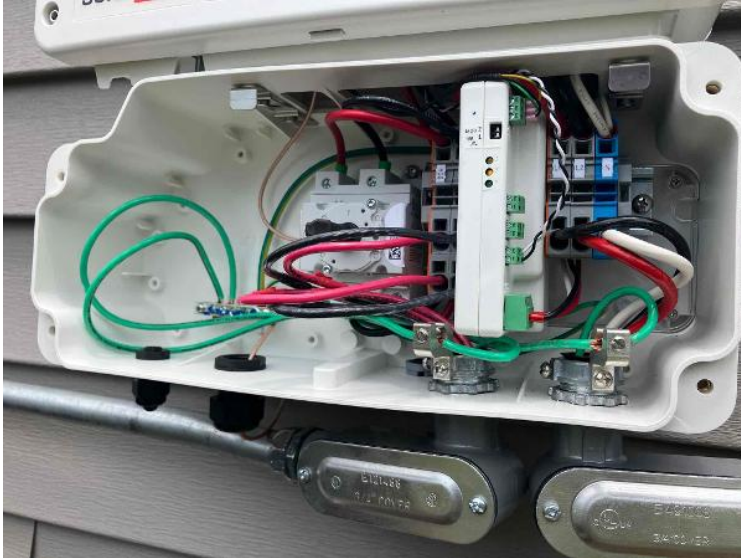
Electrical Installation / Show All Completed Wiring and Terminations for Each BOS Component
