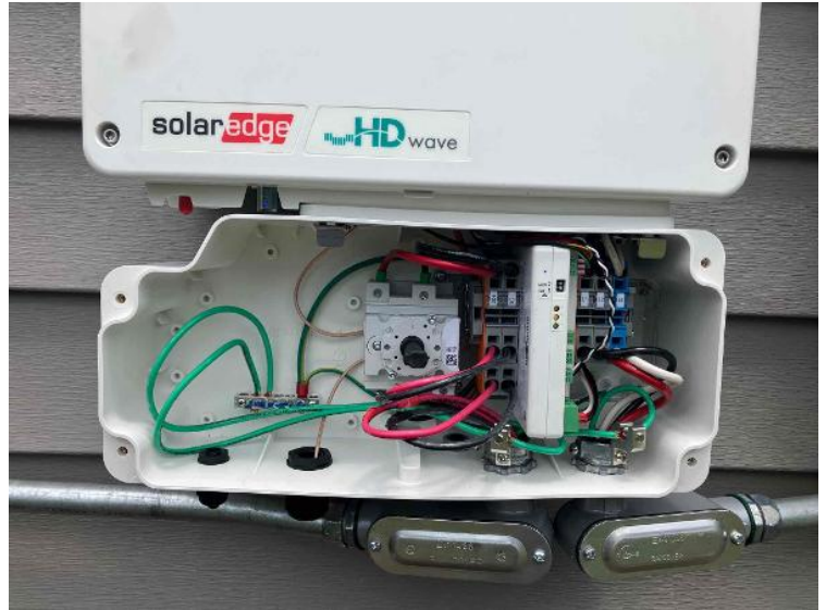
Electrical Installation / Show All Completed Wiring and Terminations for Each BOS Component
