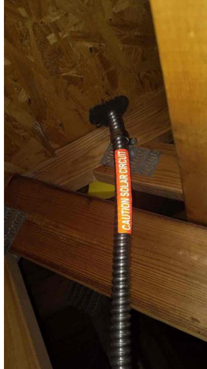
Rooftop Installation / Overall Conduit Run, Between Arrays, Attic Runs Included, Down To BOS
