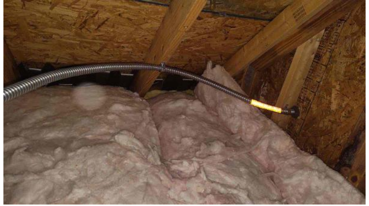
Rooftop Installation / Overall Conduit Run, Between Arrays, Attic Runs Included, Down To BOS
