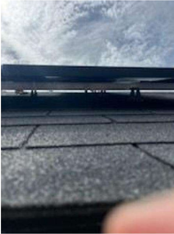
Roof Photos (All Photos with a * by them are required for panel pay bonus) / ALL Array(s) Wire Management (show that all conductors are neatly managed and clear of roof surface under all parts of each array)
