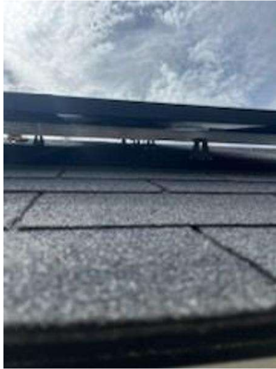
Roof Photos (All Photos with a * by them are required for panel pay bonus) / ALL Array(s) Wire Management (show that all conductors are neatly managed and clear of roof surface under all parts of each array)
