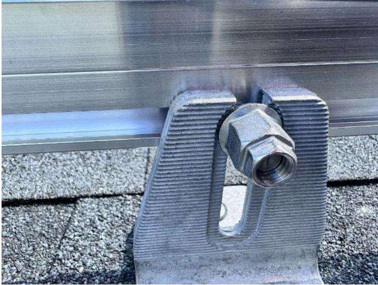
Roof Photos (All Photos with a * by them are required for panel pay bonus) / Show Mounting Points, and Show Flashing with Sealant.
