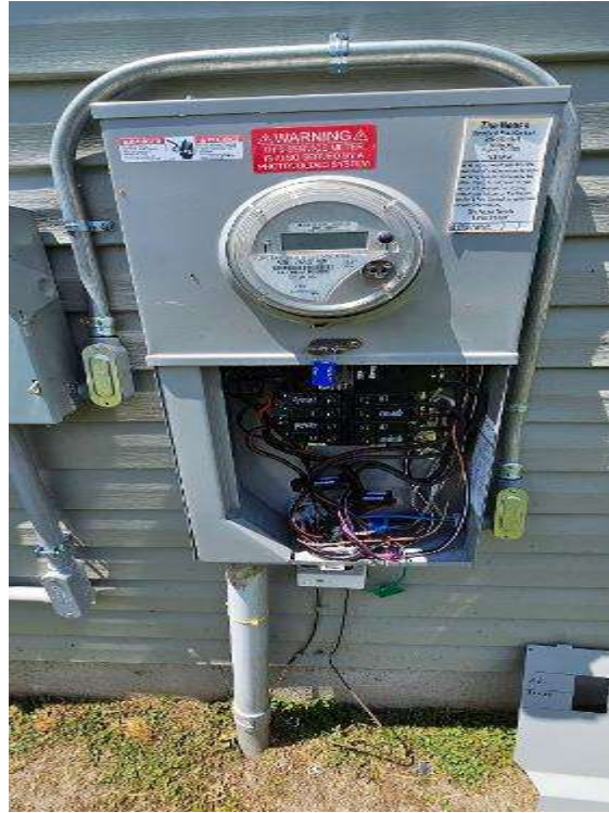
Electrical Photos (All Photos with a * by them are required for panel pay bonus) / All Electrical Equipment Interiors (show internal wiring. one pic per equipment)
