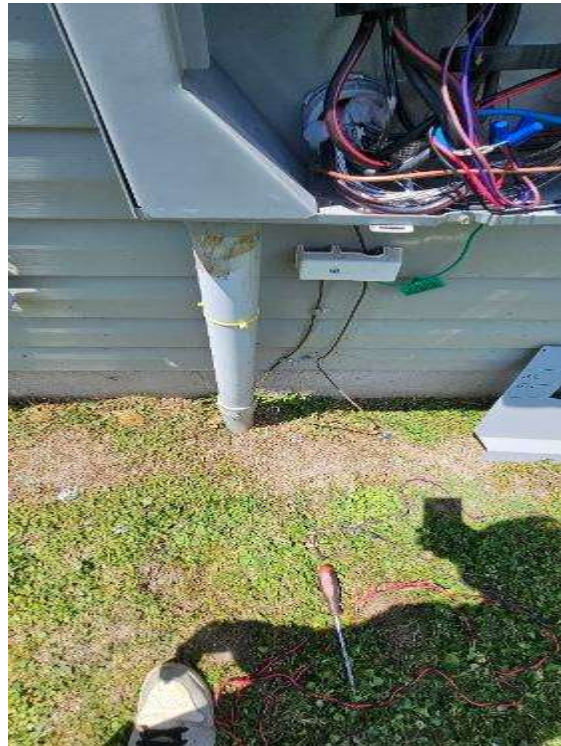
Electrical Photos (All Photos with a * by them are required for panel pay bonus) / GEC Path to ground. (Show from Ground rod or Ufer. Several Pictures.)
