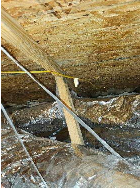
Electrical Photos (All Photos with a * by them are required for panel pay bonus) / Internal Conduit Runs. Flex Runs, Attic Runs, Basement runs.
