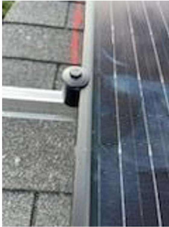
Roof Photos (All Photos with a * by them are required for panel pay bonus) / Uplclose photos of Mids and Ends
