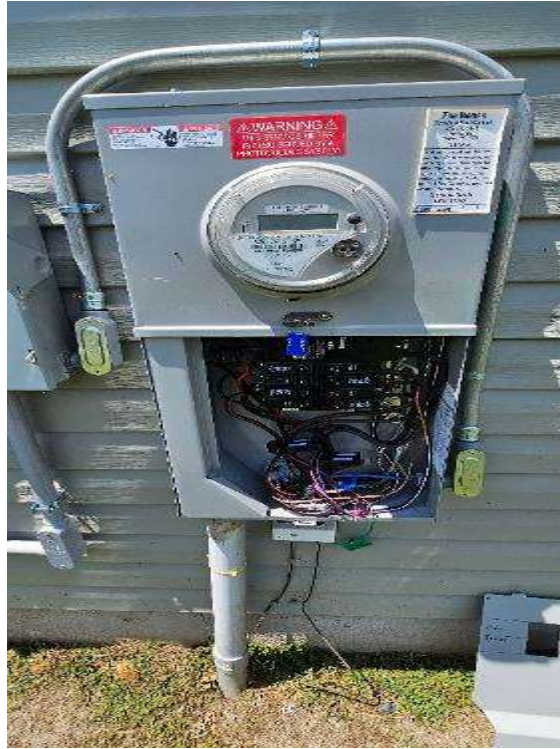
Electrical Photos (All Photos with a * by them are required for panel pay bonus) / EGC path through equipment to main. (Show Grounding in every piece of equipment)
