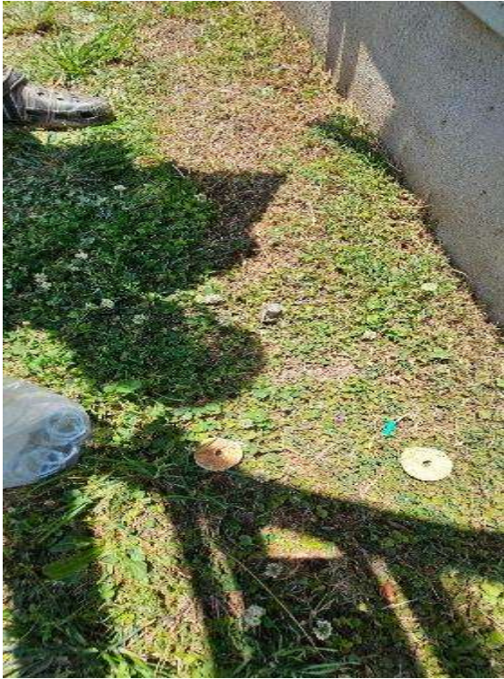
Electrical Photos (All Photos with a * by them are required for panel pay bonus) / GEC Path to ground. (Show from Ground rod or Ufer. Several Pictures.)
