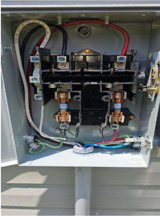
Electrical Photos (All Photos with a * by them are required for panel pay bonus) / All Electrical Equipment Interiors (show internal wiring. one pic per equipment)
