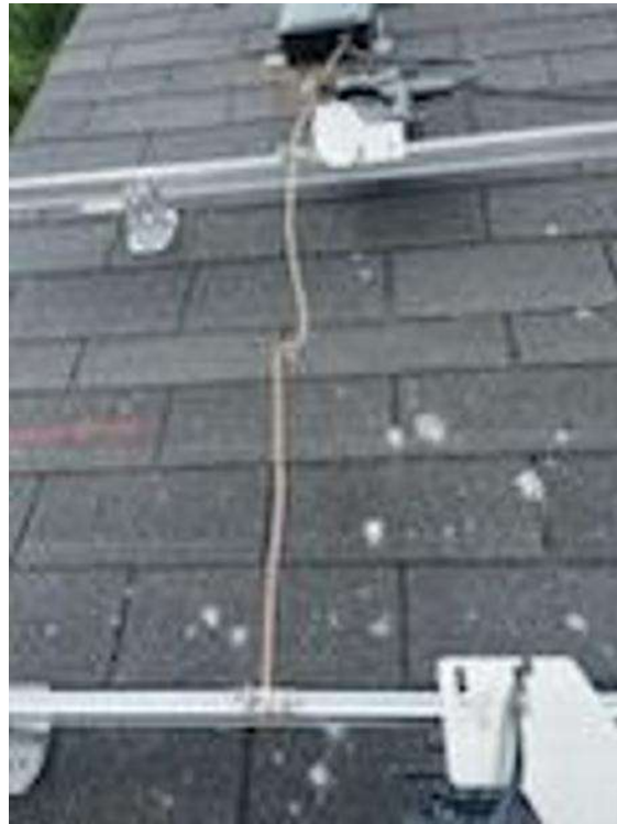
Roof Photos (All Photos with a * by them are required for panel pay bonus) / Array(s) Grounding Paths on rails. Picture of the ground on the racking (or railless grounding)
