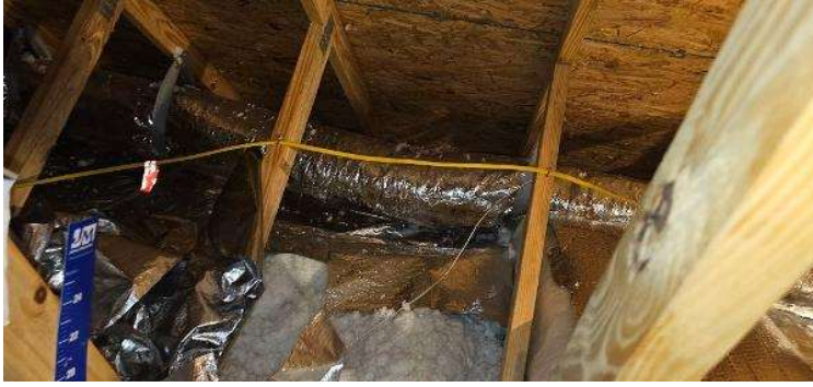
Electrical Photos (All Photos with a * by them are required for panel pay bonus) / Internal Conduit Runs. Flex Runs, Attic Runs, Basement runs.
