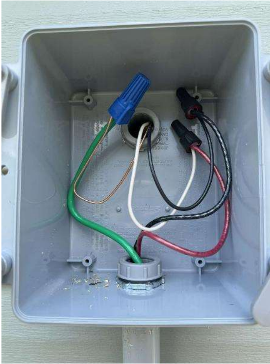
Electrical Photos (All Photos with a * by them are required for panel pay bonus) / All Electrical Equipment Interiors (show internal wiring. one pic per equipment)
