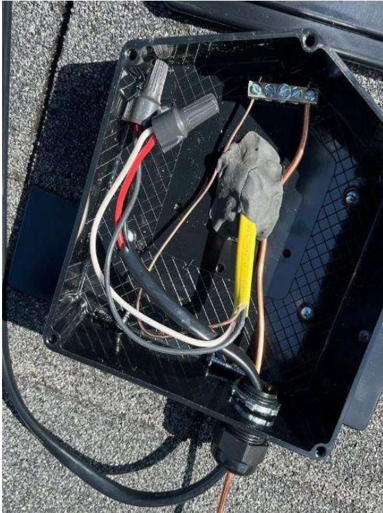
Roof Photos (All Photos with a * by them are required for panel pay bonus) / ALL Junction box interiors (wet rated wire nuts only, no MC4s)
