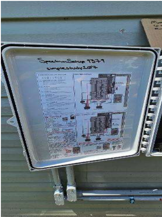
Electrical Photos (All Photos with a * by them are required for panel pay bonus) / Inverter Label (Label, or all labels if multiple showing serial number, etc)
