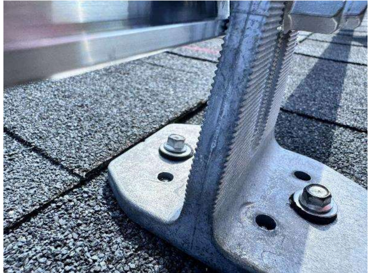
Roof Photos (All Photos with a * by them are required for panel pay bonus) / Up close Roof Penetrations (Show Method of drilled penetrations)
