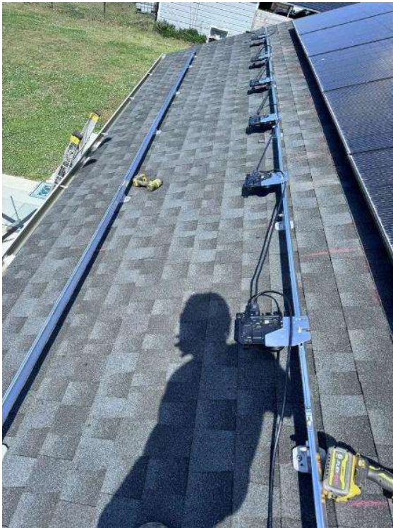
Roof Photos (All Photos with a * by them are required for panel pay bonus) / All Array(s) (Without Panels, show racking type used) ONE PHOTO PER ARRAY
