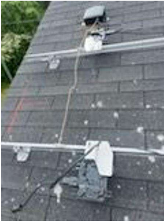
Roof Photos (All Photos with a * by them are required for panel pay bonus) / Uplclose photos of Rack Grounding
