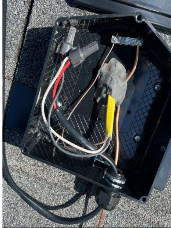
Roof Photos (All Photos with a * by them are required for panel pay bonus) / Show Soladeck Installation with sealant.
