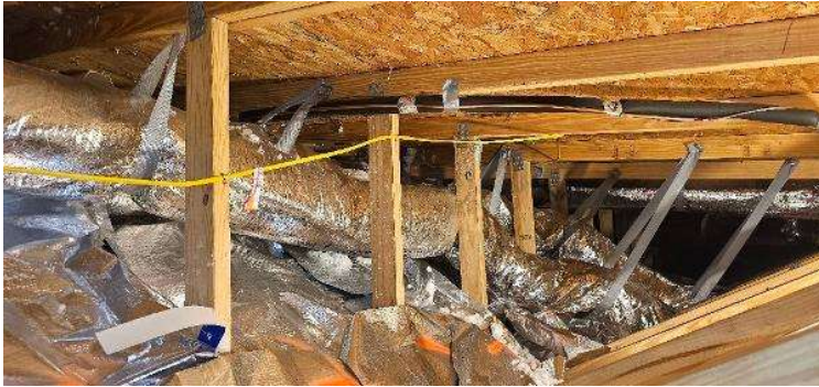
Electrical Photos (All Photos with a * by them are required for panel pay bonus) / Internal Conduit Runs. Flex Runs, Attic Runs, Basement runs.
