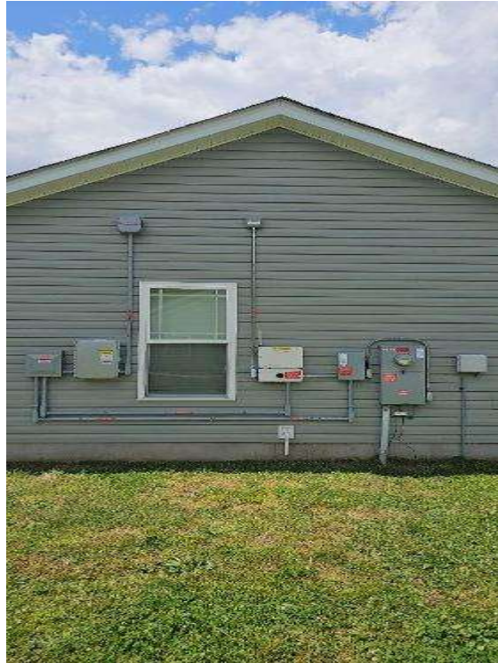
Electrical Photos (All Photos with a * by them are required for panel pay bonus) / All Electrical Warning Labels (Show them installed on equipment)
