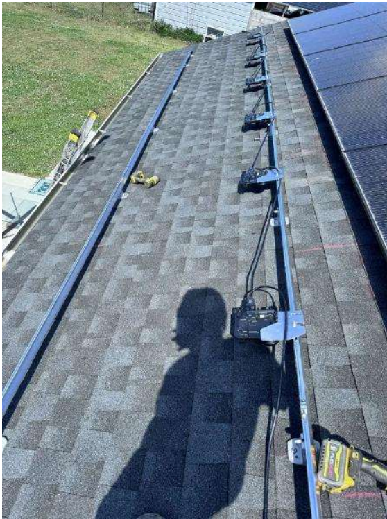
Roof Photos (All Photos with a * by them are required for panel pay bonus) / Pre-Install damage? Show bad roof boots, torn shingles, damaged gutters, etc.
