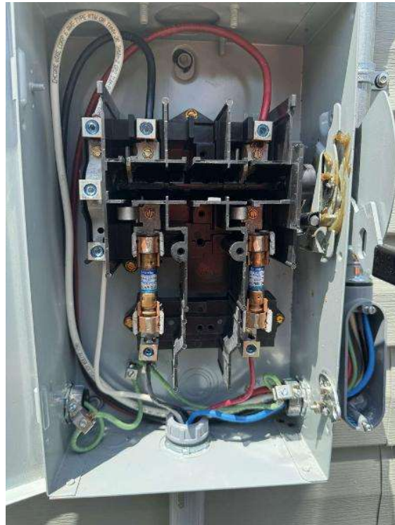
Electrical Photos (All Photos with a * by them are required for panel pay bonus) / All Electrical Equipment Interiors (show internal wiring. one pic per equipment)
