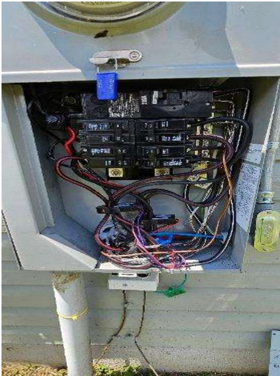
Electrical Photos (All Photos with a * by them are required for panel pay bonus) / EGC path through equipment to main. (Show Grounding in every piece of equipment)
