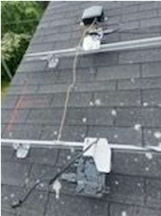
Roof Photos (All Photos with a * by them are required for panel pay bonus) / Array(s) Grounding Paths on rails. Picture of the ground on the racking (or railless grounding)
