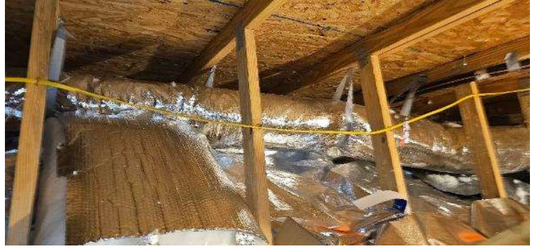
Electrical Photos (All Photos with a * by them are required for panel pay bonus) / Internal Conduit Runs. Flex Runs, Attic Runs, Basement runs.
