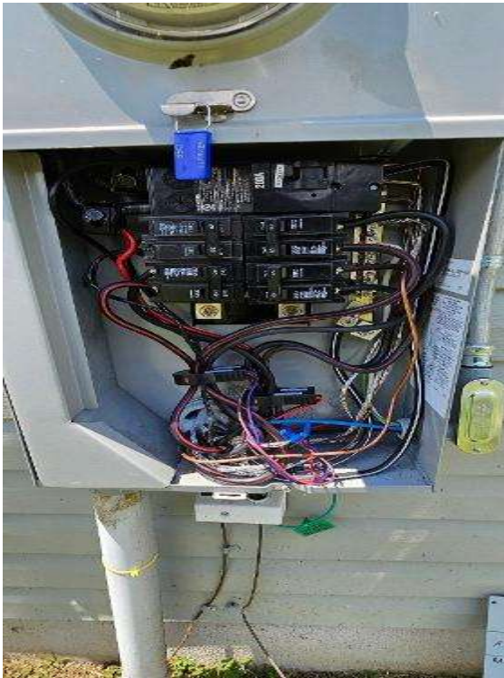
Electrical Photos (All Photos with a * by them are required for panel pay bonus) / All Electrical Equipment Interiors (show internal wiring. one pic per equipment)
