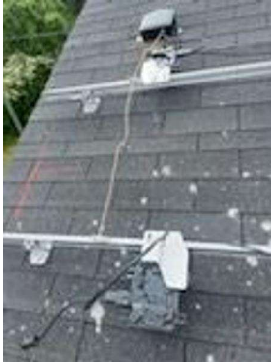
Roof Photos (All Photos with a * by them are required for panel pay bonus) / Every 2' of Grounding before panels
