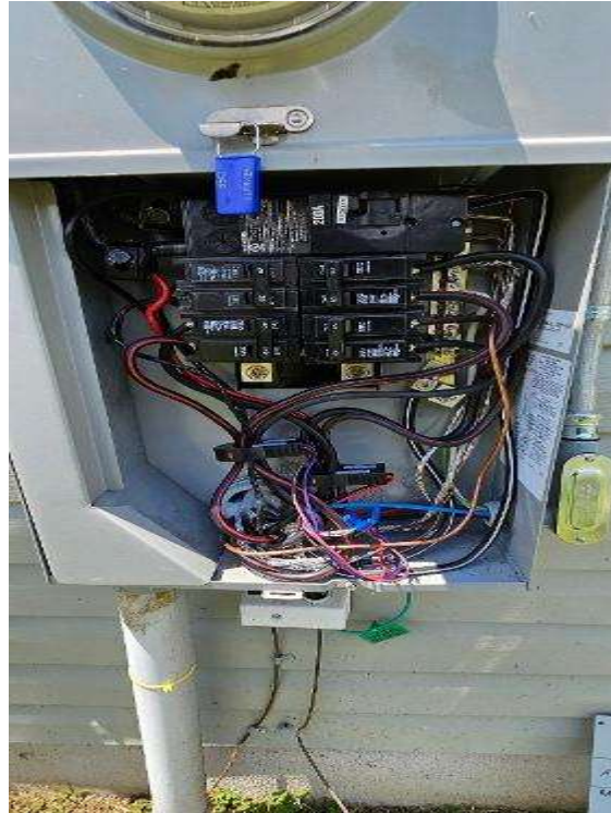
Electrical Photos (All Photos with a * by them are required for panel pay bonus) / Main Panel Label, Main Breaker Size, PV Breaker and Main Panel Interior (ONE PIC EACH ITEM)
