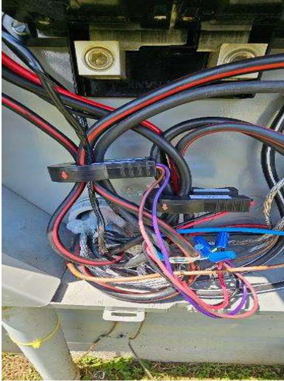
Electrical Photos (All Photos with a * by them are required for panel pay bonus) / CT's Placement in Panel
