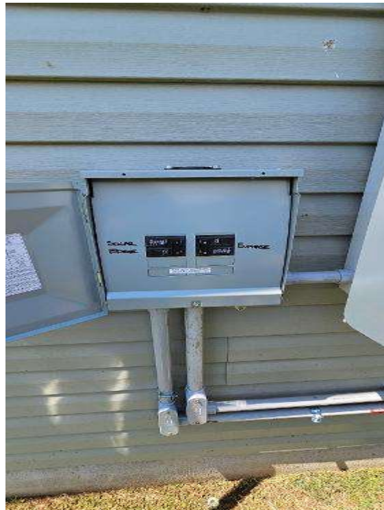
Electrical Photos (All Photos with a * by them are required for panel pay bonus) / Main Panel Label, Main Breaker Size, PV Breaker and Main Panel Interior (ONE PIC EACH ITEM)
