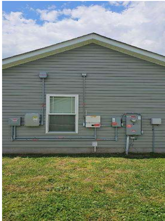
Electrical Photos (All Photos with a * by them are required for panel pay bonus) / All Electrical Equipment On Wall ( All of the electrical equipment hung, in ONE picture)
