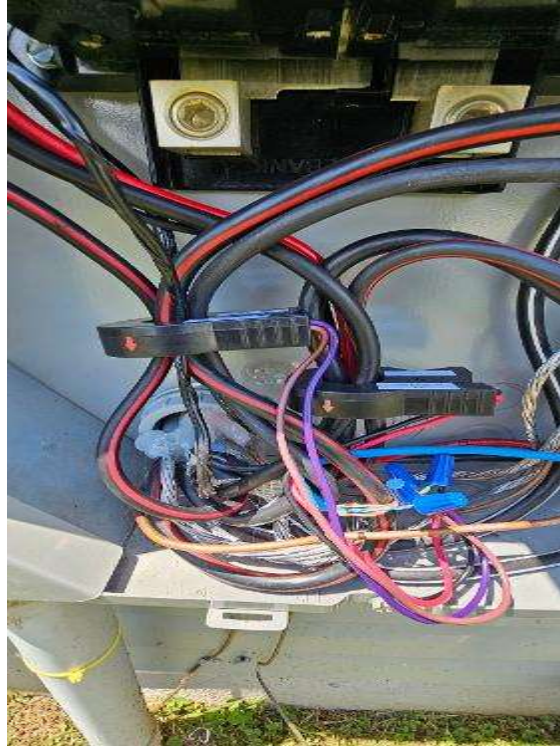
Electrical Photos (All Photos with a * by them are required for panel pay bonus) / CT's Direction. (Show both arrow directions, clearly)
