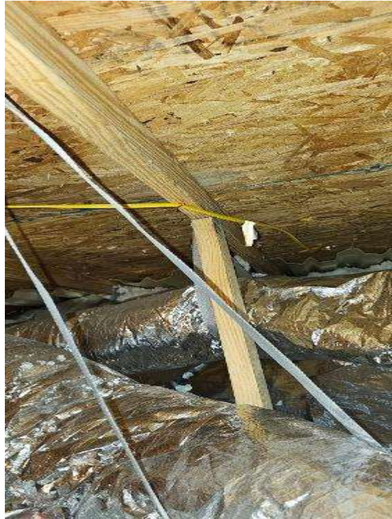
Electrical Photos (All Photos with a * by them are required for panel pay bonus) / Internal Conduit Runs. Flex Runs, Attic Runs, Basement runs.
