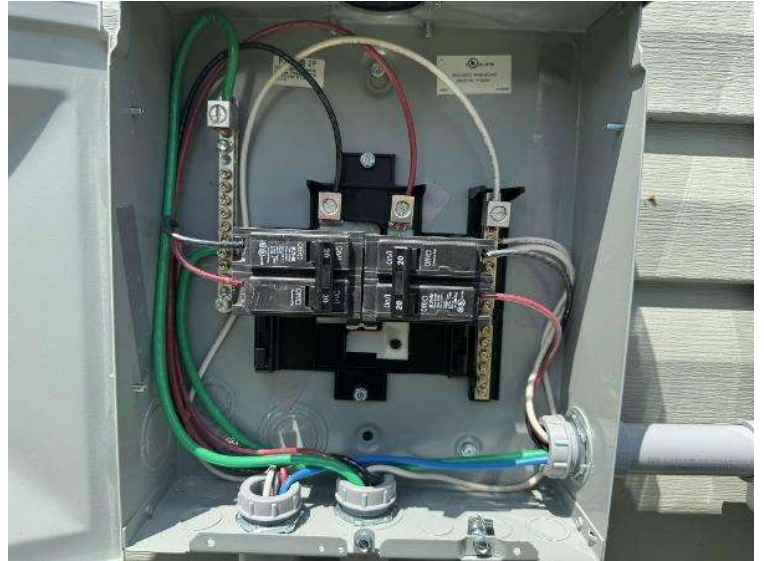
Electrical Photos (All Photos with a * by them are required for panel pay bonus) / All Electrical Equipment Interiors (show internal wiring. one pic per equipment)
