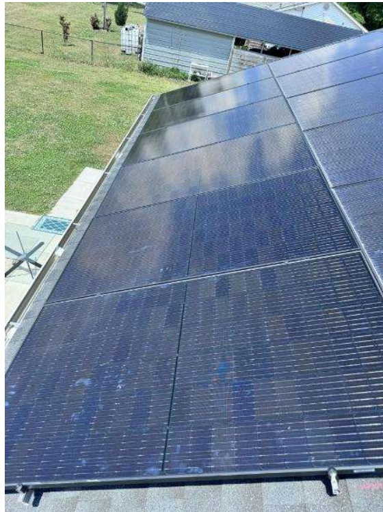
Roof Photos (All Photos with a * by them are required for panel pay bonus) / All Roof Top Conduit Paths and Supports (show path of conduit and conduit supports, properly flashed and fully installed)
