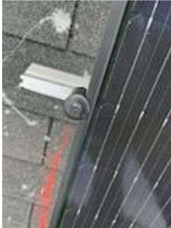
Roof Photos (All Photos with a * by them are required for panel pay bonus) / Uplclose photos of Mids and Ends
