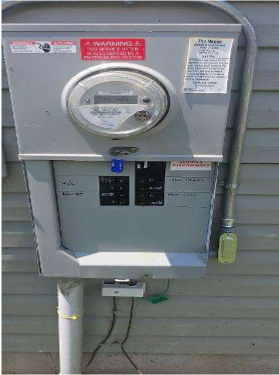
Electrical Photos (All Photos with a * by them are required for panel pay bonus) / Main Panel Label, Main Breaker Size, PV Breaker and Main Panel Interior (ONE PIC EACH ITEM)
