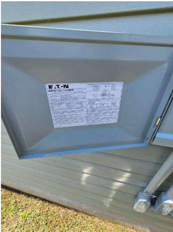
Electrical Photos (All Photos with a * by them are required for panel pay bonus) / Main Panel Label, Main Breaker Size, PV Breaker and Main Panel Interior (ONE PIC EACH ITEM)
