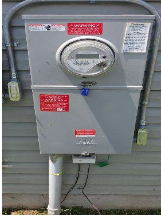
Electrical Photos (All Photos with a * by them are required for panel pay bonus) / Main Panel Label, Main Breaker Size, PV Breaker and Main Panel Interior (ONE PIC EACH ITEM)
