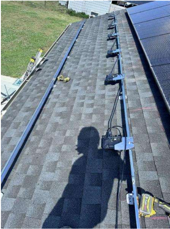
Roof Photos (All Photos with a * by them are required for panel pay bonus) / Every 2' of home runs and wire management
