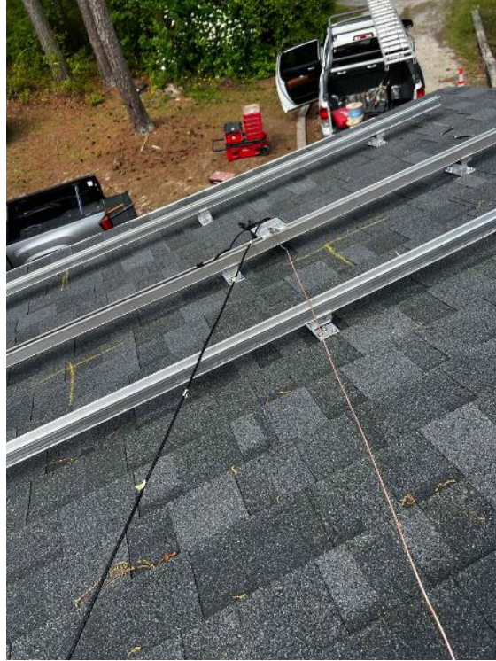
Array / Grounding: 1) Take an up close photo of the rail bonding lug along with panned out photos of the entire ground wire.
