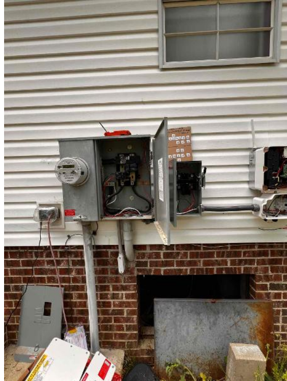
Electrical / Main Service Panel - Overall photo of entire box after interconnection
