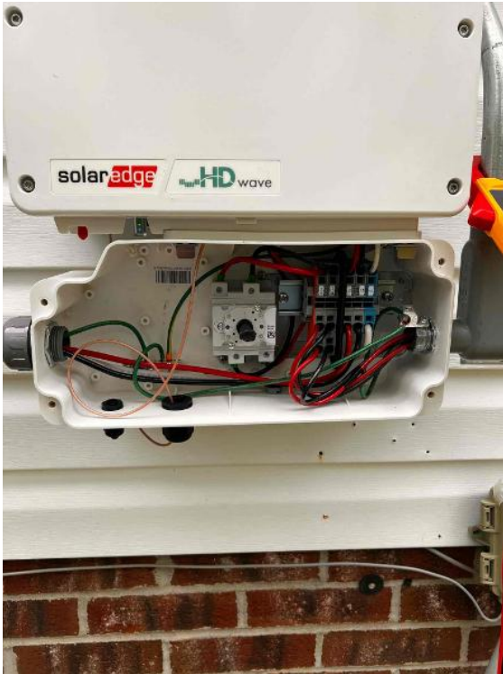
Electrical / PV Inverter or IQ Combiner - Take photo of open PV inverter or IQ Combiner showing all components installed, wiring connections, and nameplate.
