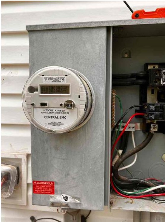
Electrical / Utility Meter - Provide legible photo of the utility meter with meter number legible
