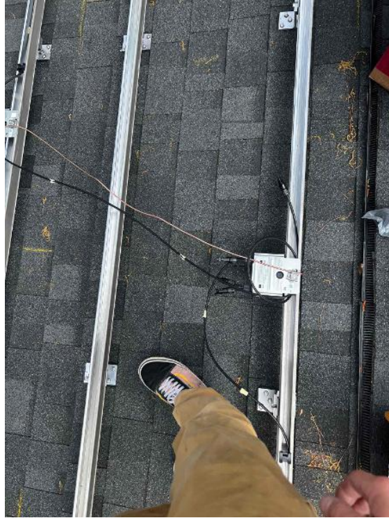
Array / Grounding: 1) Take an up close photo of the rail bonding lug along with panned out photos of the entire ground wire.
