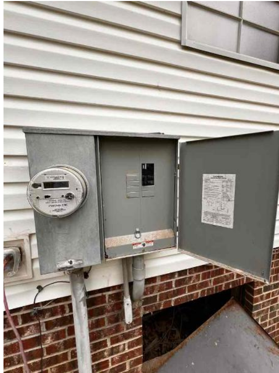
Electrical / Utility Meter - Provide legible photo of the utility meter with meter number legible
