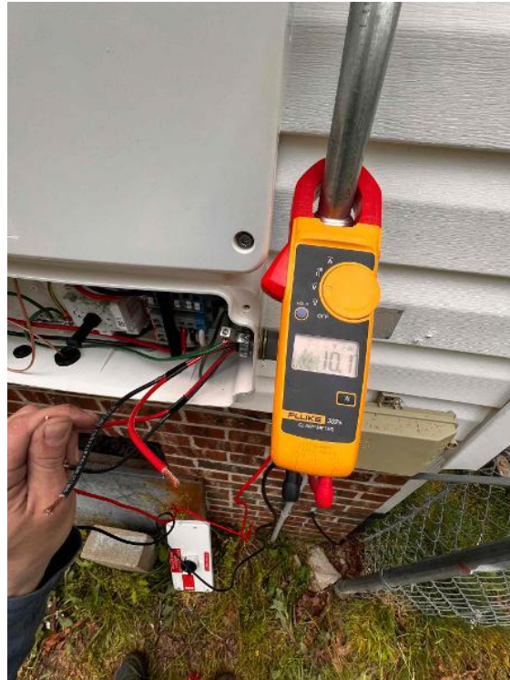
Electrical / PV Inverter or IQ Combiner - Take photo of open PV inverter or IQ Combiner showing all components installed, wiring connections, and nameplate.
