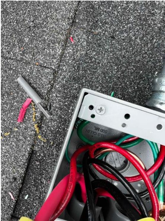
Array / PV Junction Box OPEN - All terminations, EGC path to array, attic penetration, entries & exits. (If penetrating the roof to run through the attic, the transition from attic to roof needs to be sealed with duct seal.)
