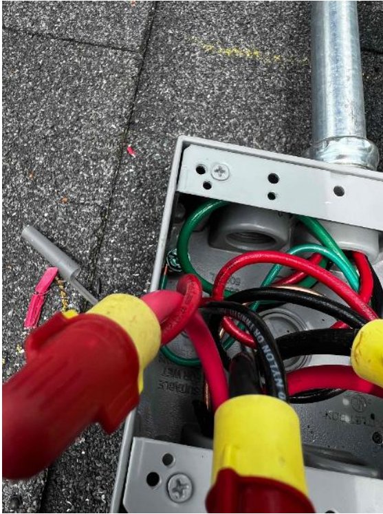
Array / PV Junction Box OPEN - All terminations, EGC path to array, attic penetration, entries & exits. (If penetrating the roof to run through the attic, the transition from attic to roof needs to be sealed with duct seal.)
