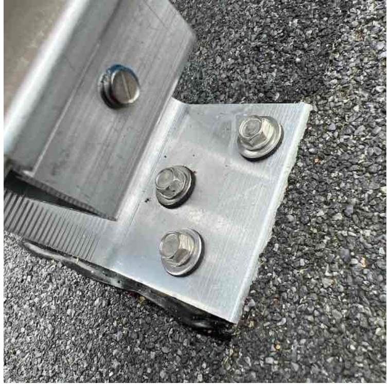
Roof Leak Prevention / Photo of at least 1 flashing with sealant applied in the correct U-shape
