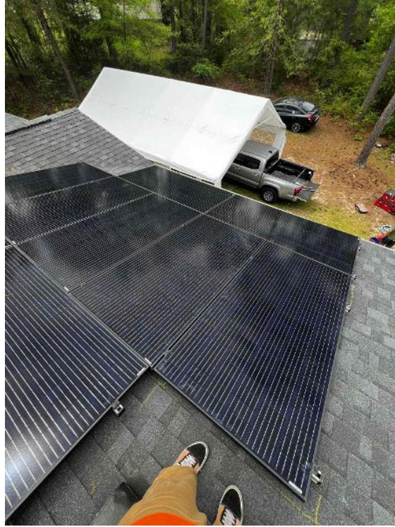
Array / Module Attachments - Need to show panels are properly secured and torqued to spec with mid clamps and end clamps.
