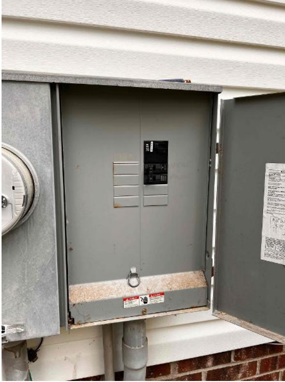
Electrical / Main Service Panel: Detailed photos of tie method with main breaker rating and backfed breaker rating clearly legible.
