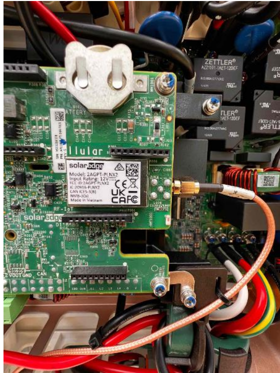
Electrical / Communication Devices Installed - Provide photos of all communication devices installed.
