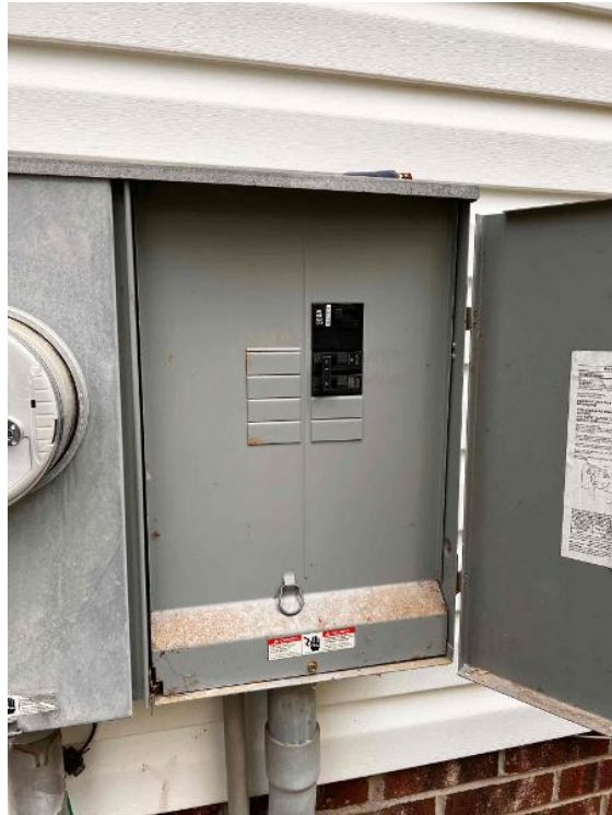
Electrical / Main Service Panel Nameplate - Take a photo of the MSP nameplate. BUSBAR RATING MUST BE LEGIBLE. THIS CAN OFTEN ONLY BE FOUND ON THE INSIDE WALL OF THE CABINET.
