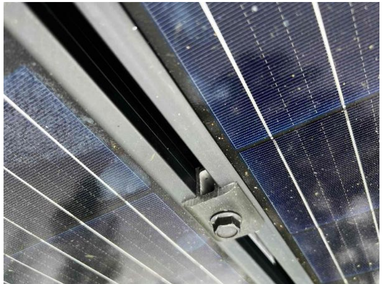
Array / Module Attachments - Need to show panels are properly secured and torqued to spec with mid clamps and end clamps.
