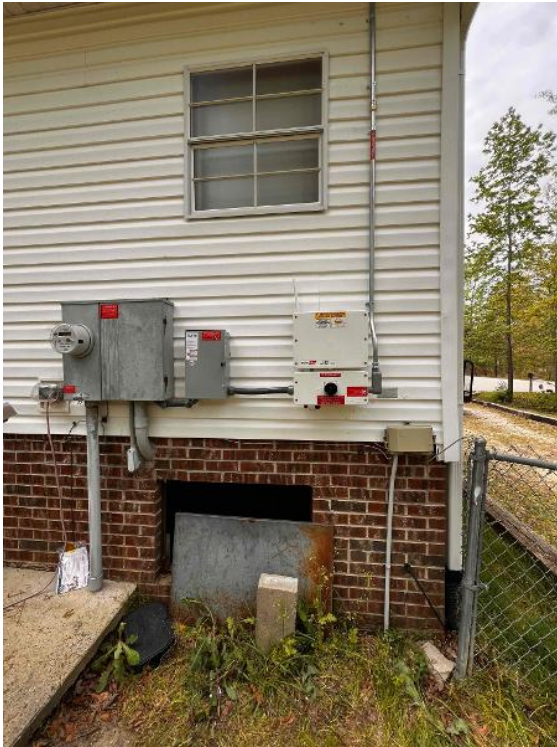
Electrical / PV Equipment - A panned out photo of all PV equipment installed and completed.
