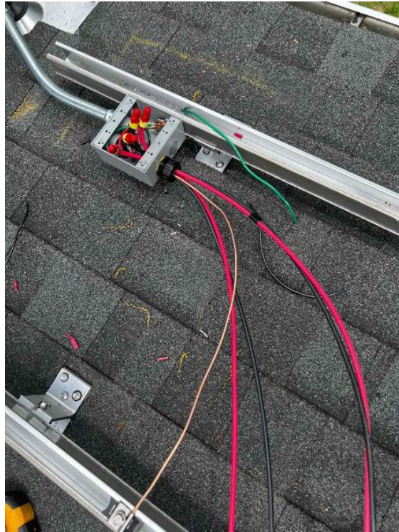
Conduit and Wire Run / Conduit Attachment - Take a close up photo of conduit attachment
