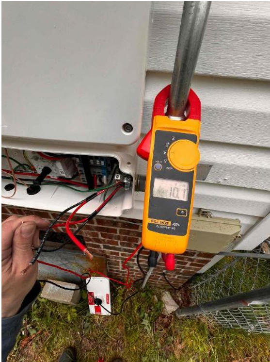
Electrical / SolarEdge Multimeter Readings: Show the Voc for each PV string, to confirm the Voc is within the expected range. Do NOT skip this step.
