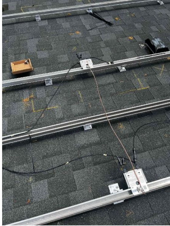
Array / Grounding: 1) Take an up close photo of the rail bonding lug along with panned out photos of the entire ground wire.
