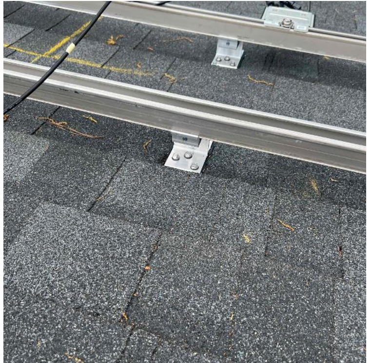
Array / Roof Attachment - Need to show the penetration/flashing sealed properly. Need multiple photos showing the correct application.
