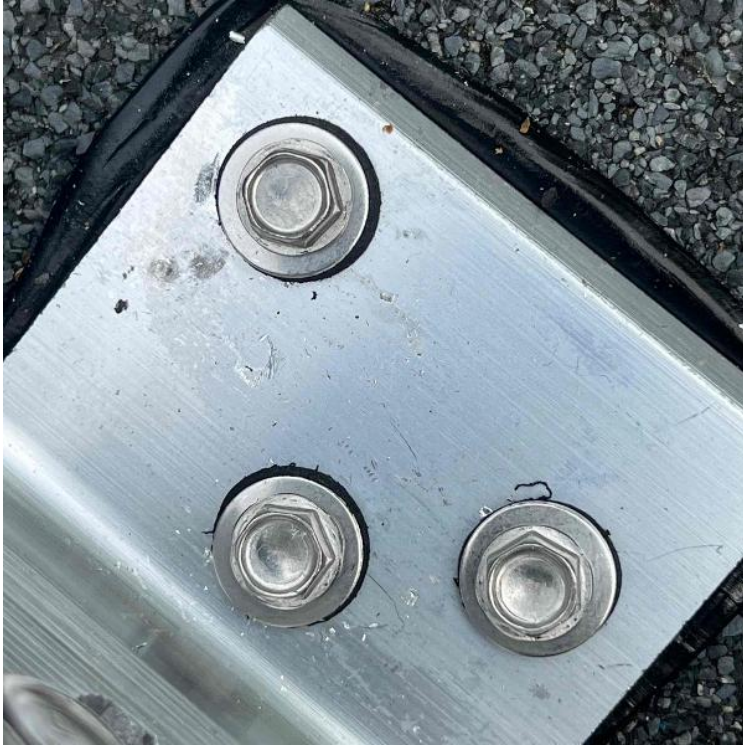
Array / Roof Attachment - Need to show the penetration/flashing sealed properly. Need multiple photos showing the correct application.
