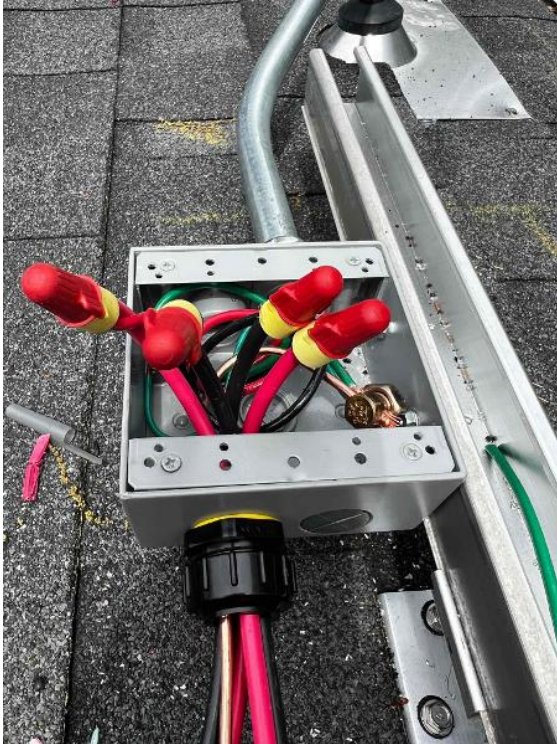
Conduit and Wire Run / Conduit Attachment - Take a close up photo of conduit attachment
