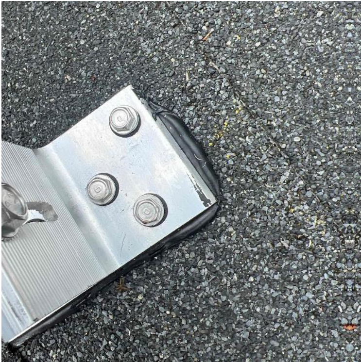
Array / Roof Attachment - Need to show the penetration/flashing sealed properly. Need multiple photos showing the correct application.
