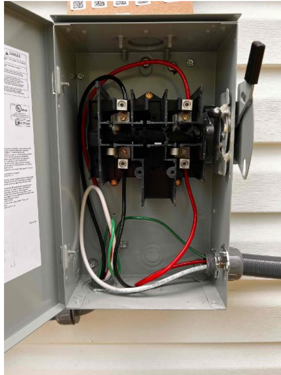
Electrical / PV System Disconnect - Photos of PV system disconnect, including fuse sizes and wire sizes.
