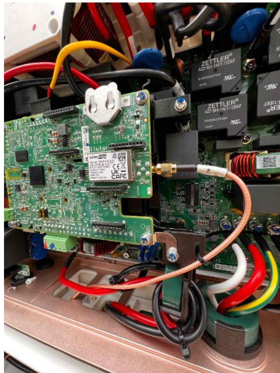
Electrical / Communication Device Serial Numbers - Take clear photos of the communication device serial numbers on site.
