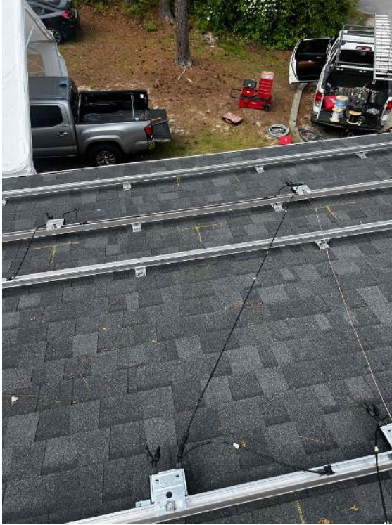
Array / Grounding: 1) Take an up close photo of the rail bonding lug along with panned out photos of the entire ground wire.
