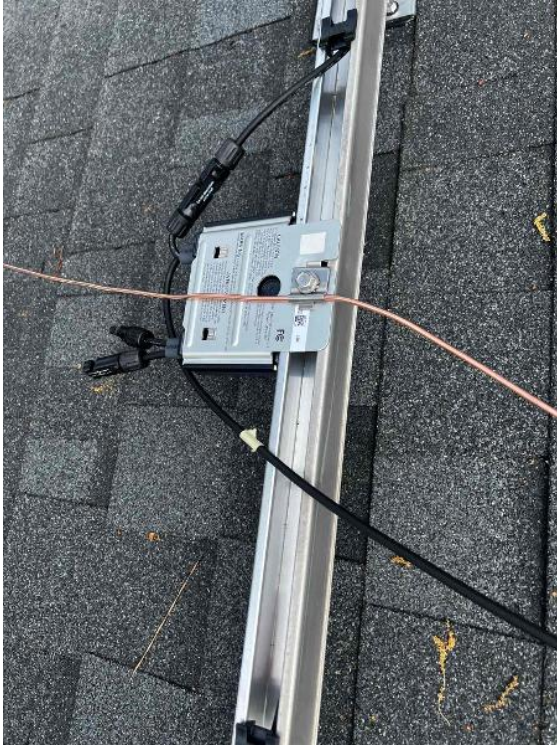
Array / Grounding: 1) Take an up close photo of the rail bonding lug along with panned out photos of the entire ground wire.
