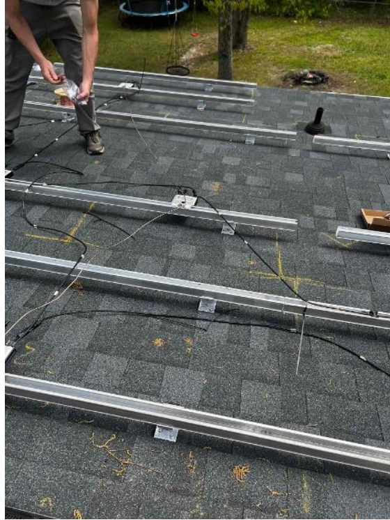
Array / Grounding: 1) Take an up close photo of the rail bonding lug along with panned out photos of the entire ground wire.
