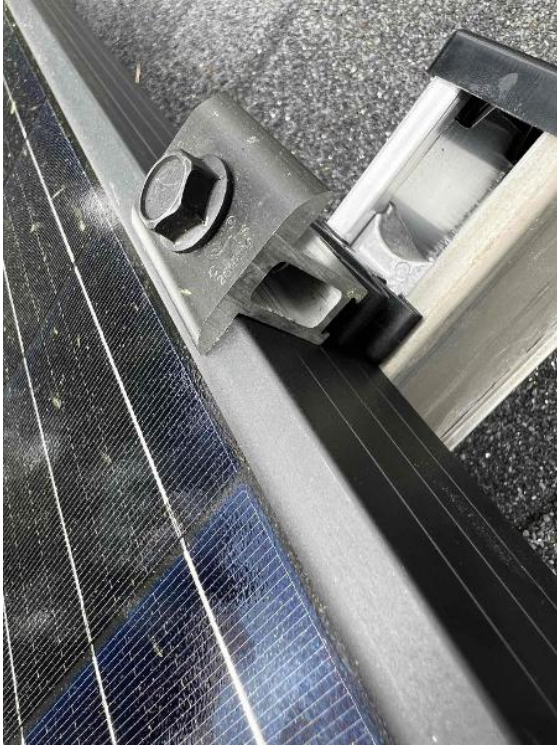
Array / Module Attachments - Need to show panels are properly secured and torqued to spec with mid clamps and end clamps.
