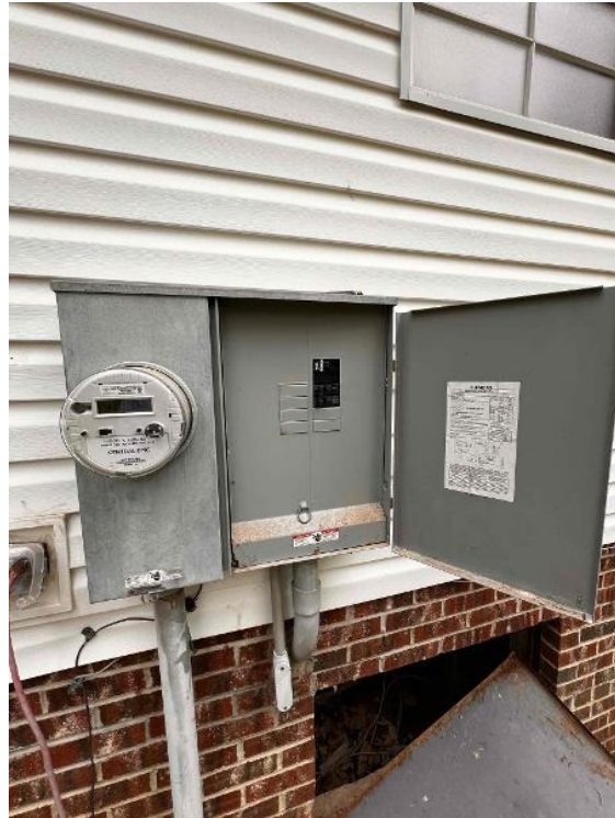
Electrical / Main Service Panel: Detailed photos of tie method with main breaker rating and backed breaker rating clearly legible.
