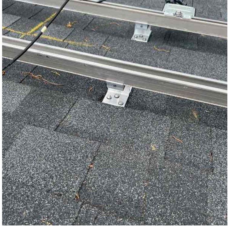
Roof Leak Prevention / Photos of any unused penetrations properly flashed and sealed with aluminum
