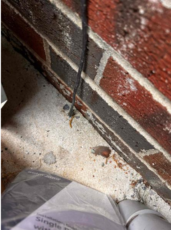
Electrical / GEC (Grounding Electrode Conductor) - Take photos of the main GEC including ground rods and acorn clamps.
