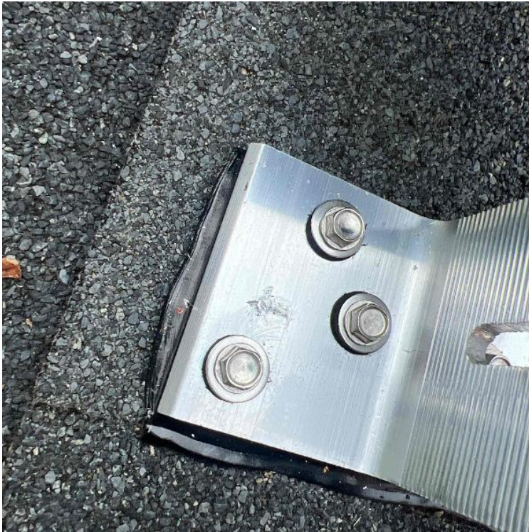
Array / Roof Attachment - Need to show the penetration/flashing sealed properly. Need multiple photos showing the correct application.
