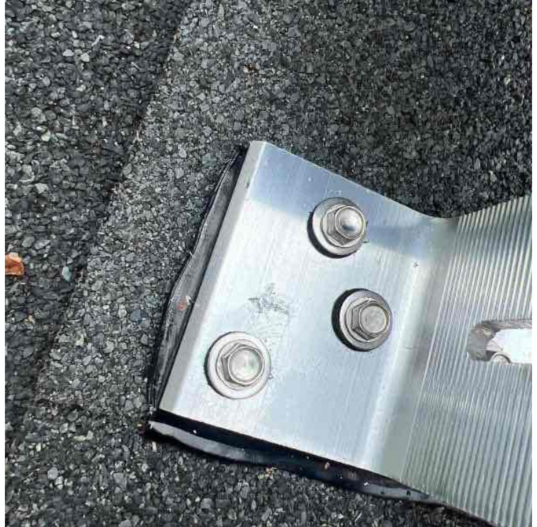
Roof Leak Prevention / Photos of any unused penetrations properly flashed and sealed with aluminum
