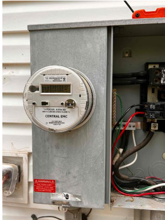
Electrical / Main Service Panel: Detailed photos of tie method with main breaker rating and backed breaker rating clearly legible.
