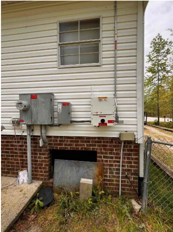
Electrical / PV Labels - photo of all PV labels installed, close up and overview (note if missing any)
