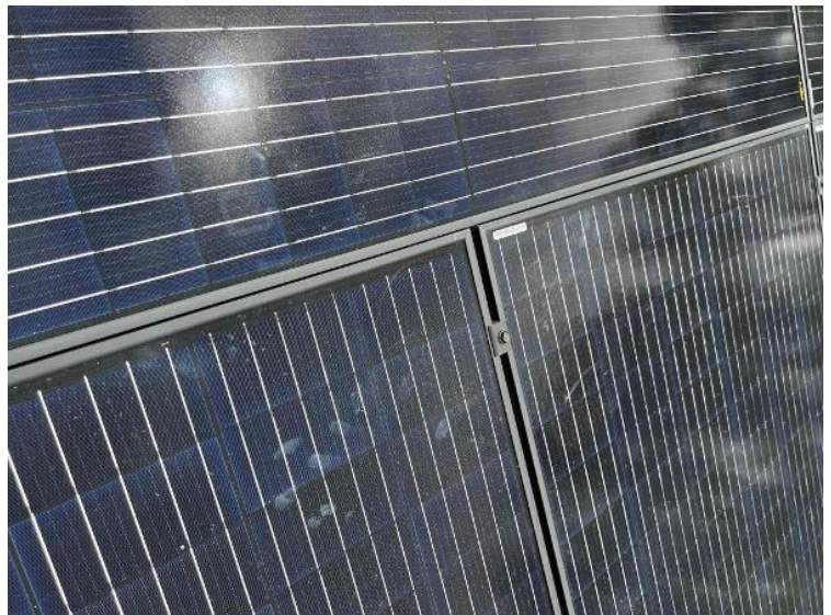
Array / Module Attachments - Need to show panels are properly secured and torqued to spec with mid clamps and end clamps.
