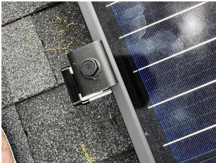
Array / Module Attachments - Need to show panels are properly secured and torqued to spec with mid clamps and end clamps.
