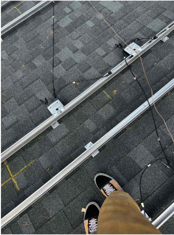
Array / Grounding: 1) Take an up close photo of the rail bonding lug along with panned out photos of the entire ground wire.
