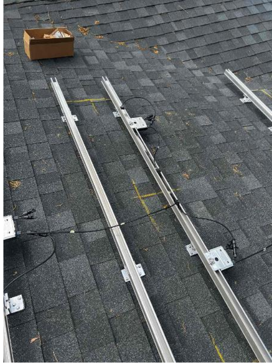
Array / Grounding: 1) Take an up close photo of the rail bonding lug along with panned out photos of the entire ground wire.
