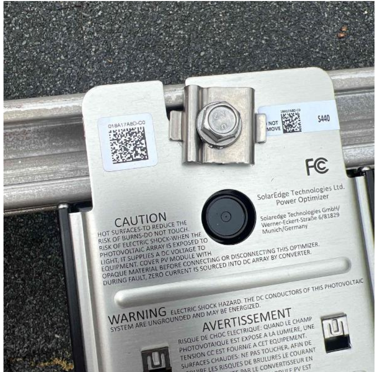
Array / MLPE (micro inverter/optimizer) serial number, must include model number as well. SOLAREEDGE OPTIMIZER MODEL NUMBERS ARE NOT VISIBLE FROM TOP DOWN VIEW
