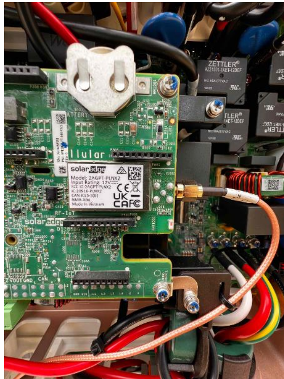
Electrical / Communication Device Serial Numbers - Take clear photos of the communication device serial numbers on site.
