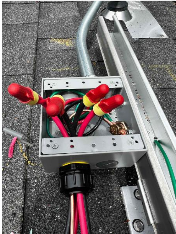
Array / PV Junction Box OPEN - All terminations, EGC path to array, attic penetration, entries & exits. (If penetrating the roof to run through the attic, the transition from attic to roof needs to be sealed with duct seal.)
