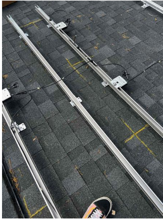
Array / Grounding: 1) Take an up close photo of the rail bonding lug along with panned out photos of the entire ground wire.
