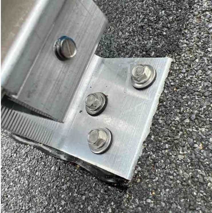
Roof Leak Prevention / Photos of any unused penetrations properly flashed and sealed with aluminum
