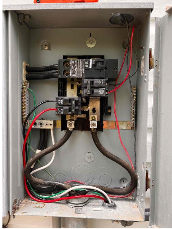
Electrical / Main Service Panel: Detailed photos of tie method with main breaker rating and backfed breaker rating clearly legible.
