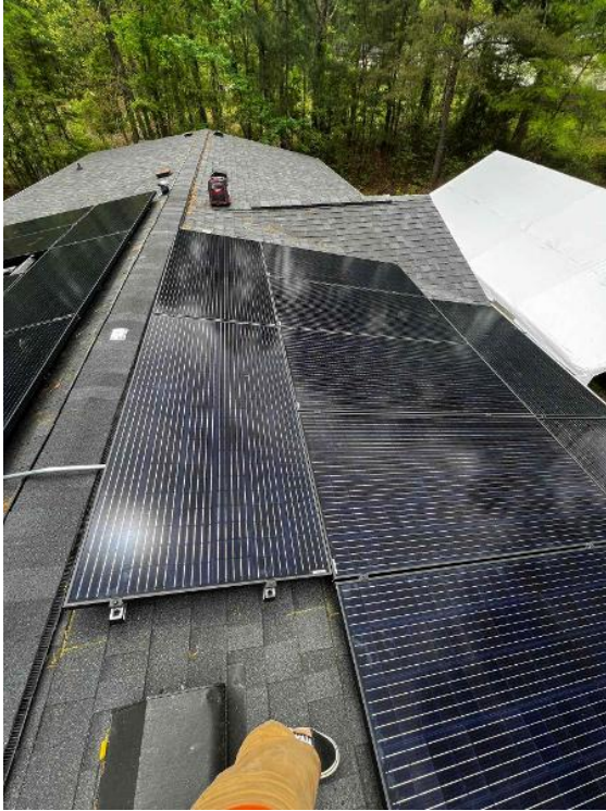
Array / Module Attachments - Need to show panels are properly secured and torqued to spec with mid clamps and end clamps.
