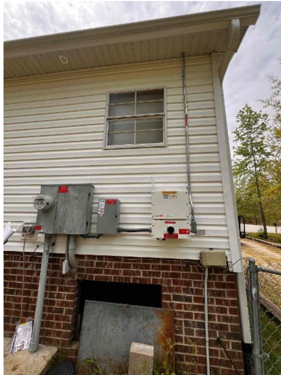
Electrical / PV Labels - photo of all PV labels installed, close up and overview (note if missing any)
