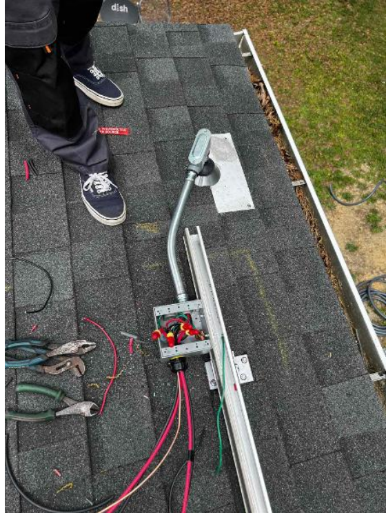
Conduit and Wire Run / Conduit Attachment - Take a close up photo of conduit attachment
