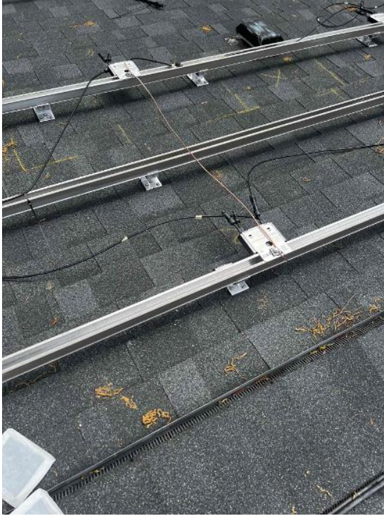
Array / Grounding: 1) Take an up close photo of the rail bonding lug along with panned out photos of the entire ground wire.
