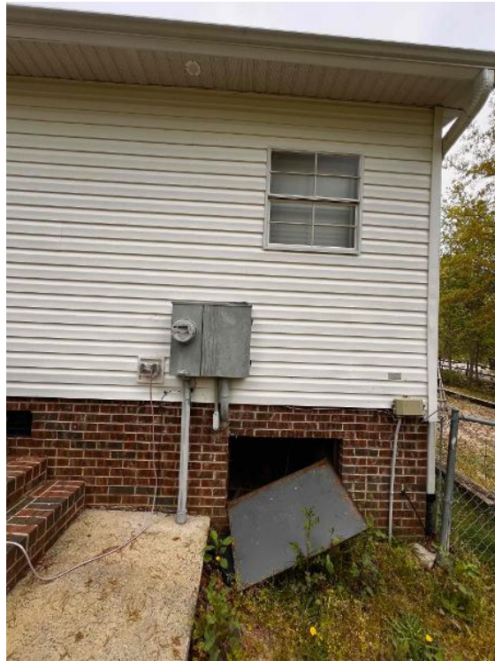
Electrical / PV Equipment - A panned out photo of all PV equipment installed and completed.
