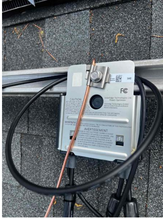
Array / Grounding: 1) Take an up close photo of the rail bonding lug along with panned out photos of the entire ground wire.
