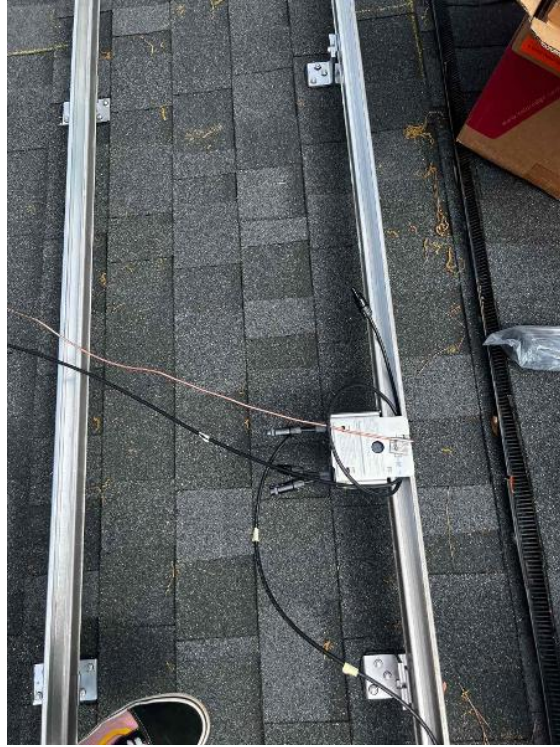
Array / Grounding: 1) Take an up close photo of the rail bonding lug along with panned out photos of the entire ground wire.
