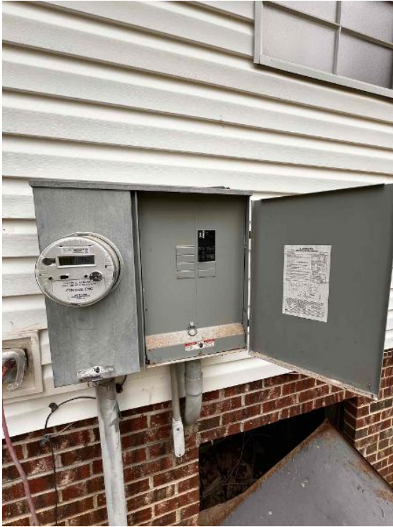
Electrical / Main Service Panel Nameplate - Take a photo of the MSP nameplate. BUSBAR RATING MUST BE LEGIBLE. THIS CAN OFTEN ONLY BE FOUND ON THE INSIDE WALL OF THE CABINET.
