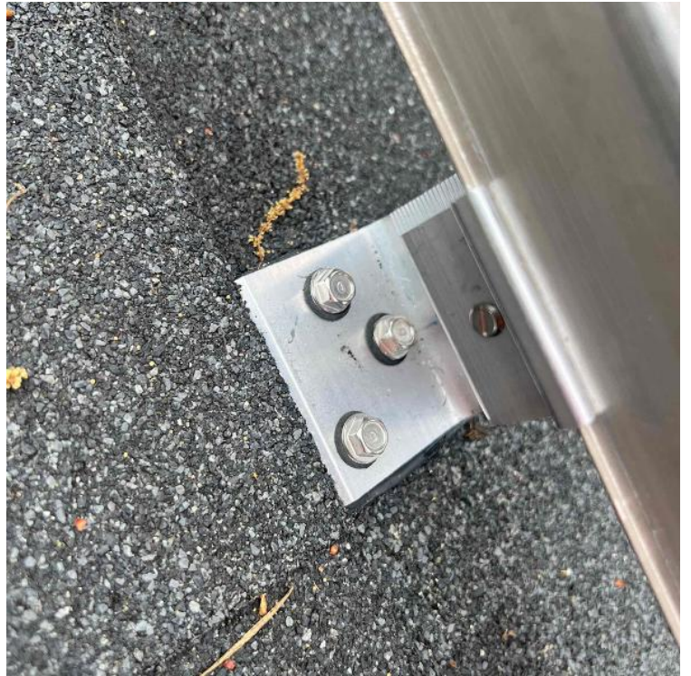
Array / Roof Attachment - Need to show the penetration/flashing sealed properly. Need multiple photos showing the correct application.
