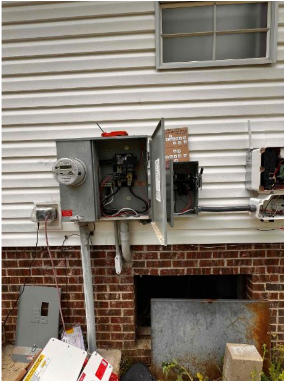
Electrical / Main Service Panel: Detailed photos of tie method with main breaker rating and backed breaker rating clearly legible.
