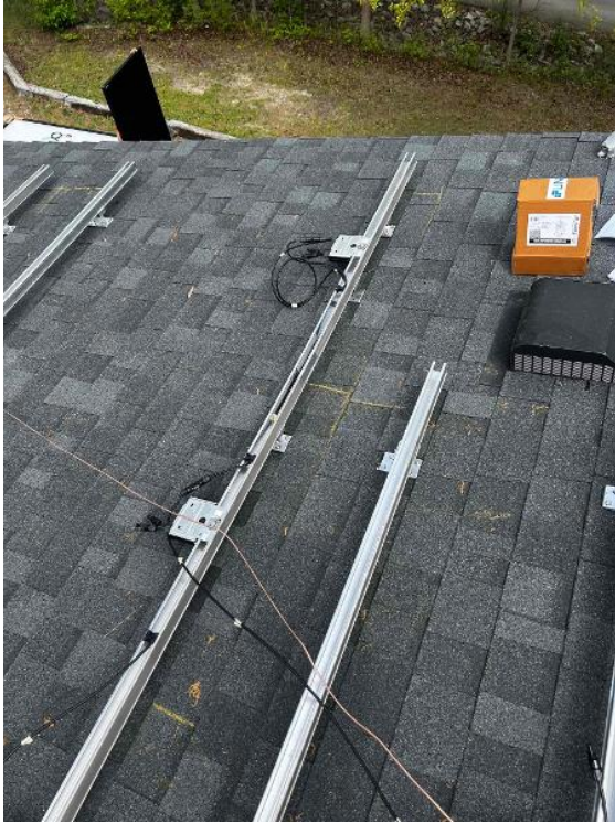
Array / Grounding: 1) Take an up close photo of the rail bonding lug along with panned out photos of the entire ground wire.
