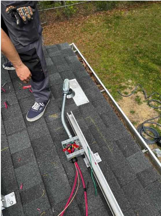
Conduit and Wire Run / Conduit Attachment - Take a close up photo of conduit attachment
