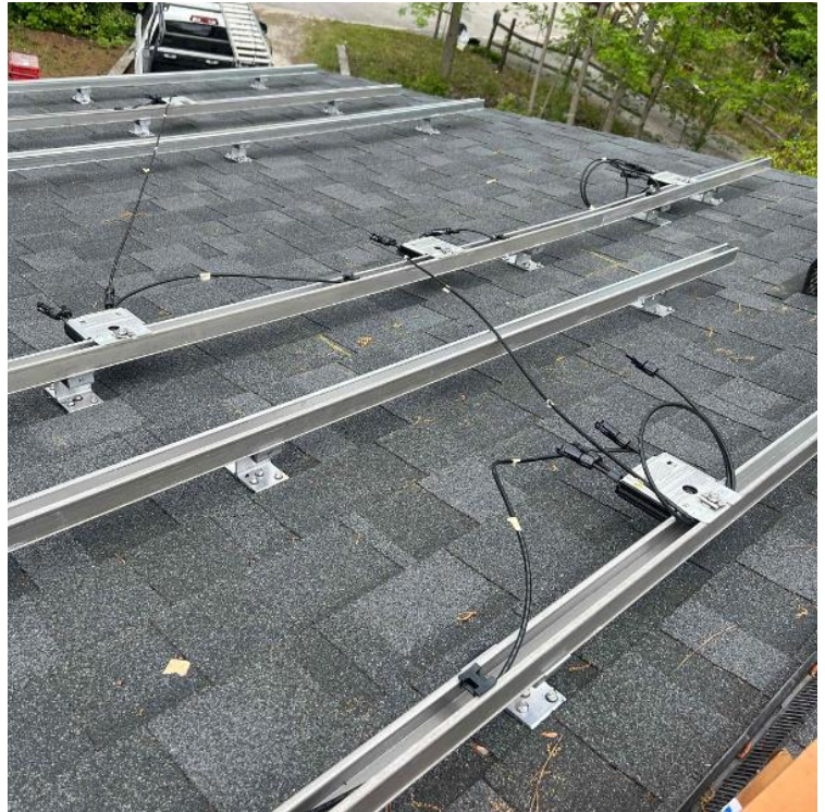
Array / Roof Attachment and Racking Layout - showing COMPLETE layouts, staggered attachments, span measurement. (2 pics per array min) If this is a tile roof get some clear photos of the tile condition before laying panels.
