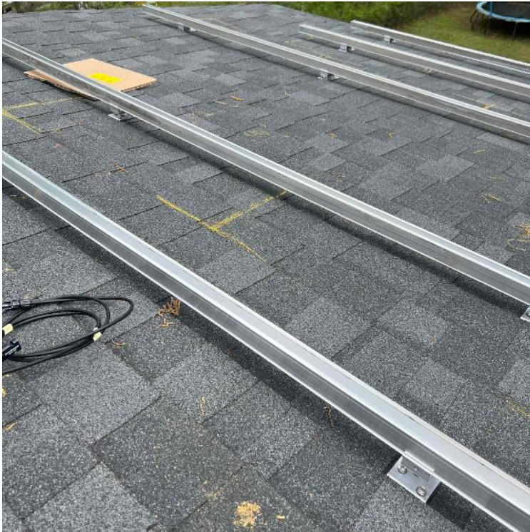
Array / Roof Attachment and Racking Layout - showing COMPLETE layouts, staggered attachments, span measurement. (2 pics per array min) If this is a tile roof get some clear photos of the tile condition before laying panels.
