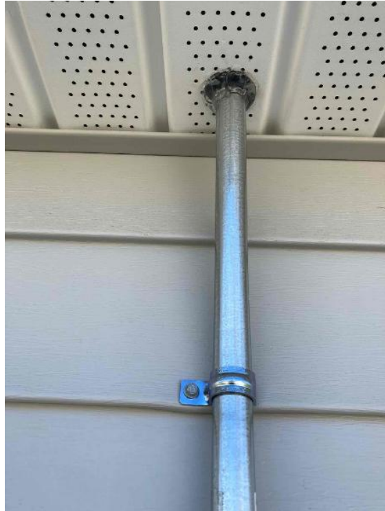
Rooftop Installation / Sealant Around Conduit Through Eave
