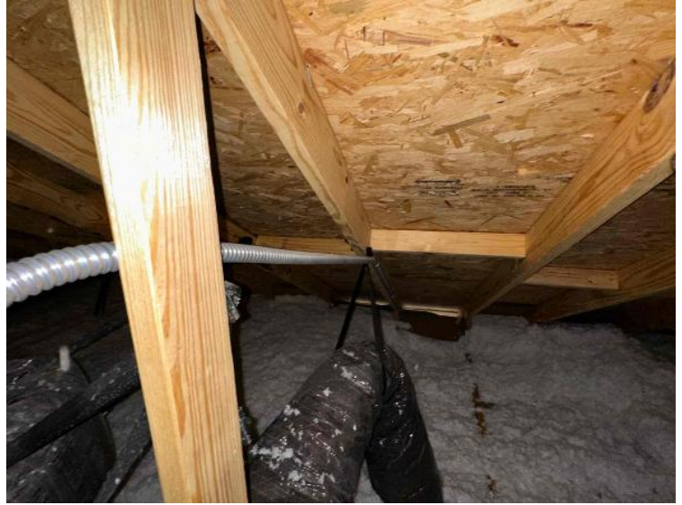
Rooftop Installation / Overall Conduit Run, Between Arrays, Attic Runs Included, Down To BOS
