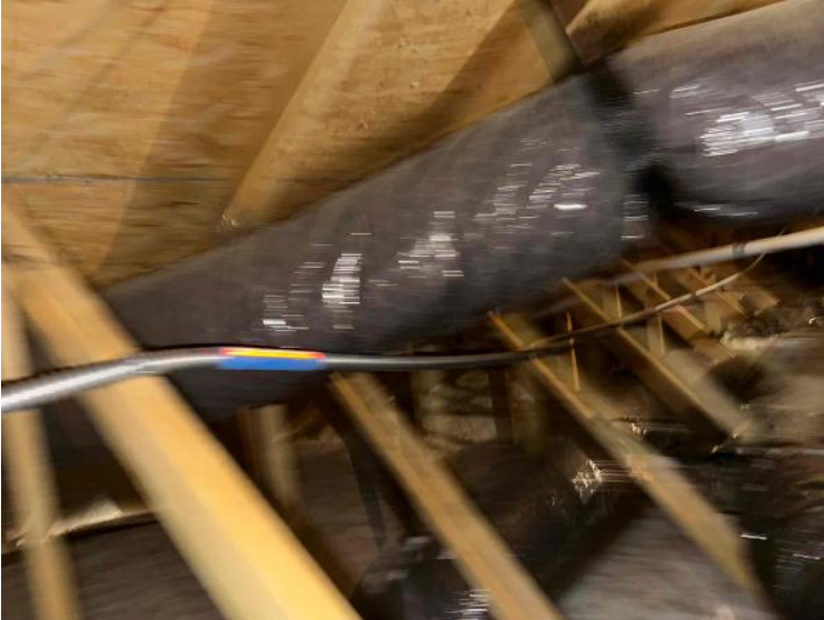
Rooftop Installation / Overall Conduit Run, Between Arrays, Attic Runs Included, Down To BOS
