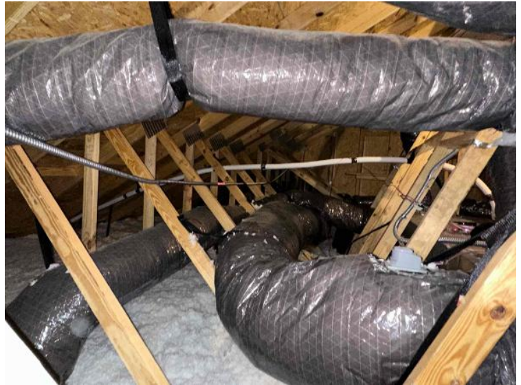
Rooftop Installation / Overall Conduit Run, Between Arrays, Attic Runs Included, Down To BOS
