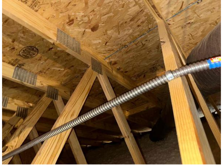
Rooftop Installation / Overall Conduit Run, Between Arrays, Attic Runs Included, Down To BOS
