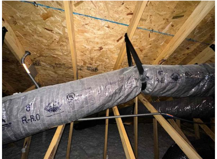
Rooftop Installation / Overall Conduit Run, Between Arrays, Attic Runs Included, Down To BOS
