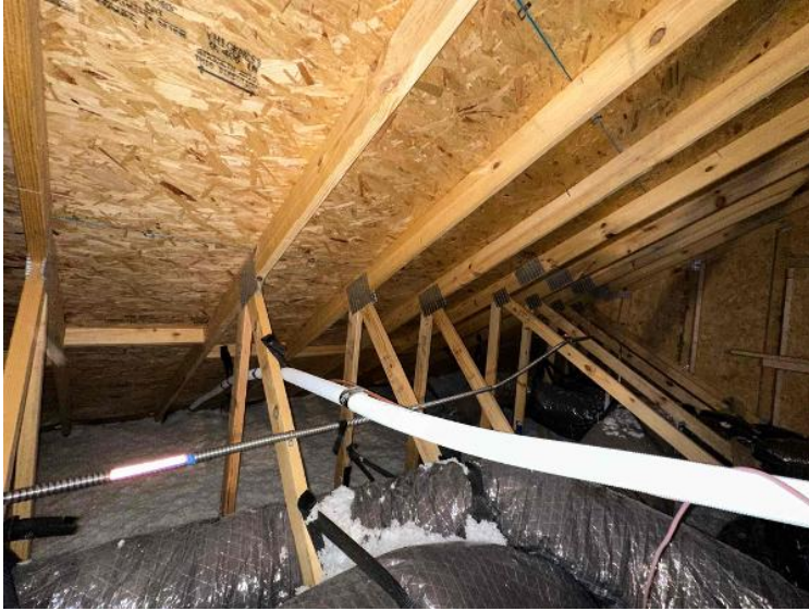
Rooftop Installation / Overall Conduit Run, Between Arrays, Attic Runs Included, Down To BOS
