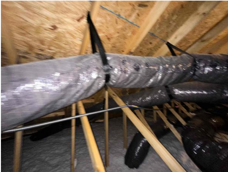
Rooftop Installation / Overall Conduit Run, Between Arrays, Attic Runs Included, Down To BOS
