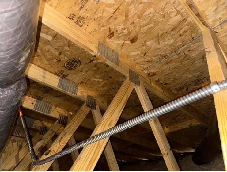
Rooftop Installation / Overall Conduit Run, Between Arrays, Attic Runs Included, Down To BOS
