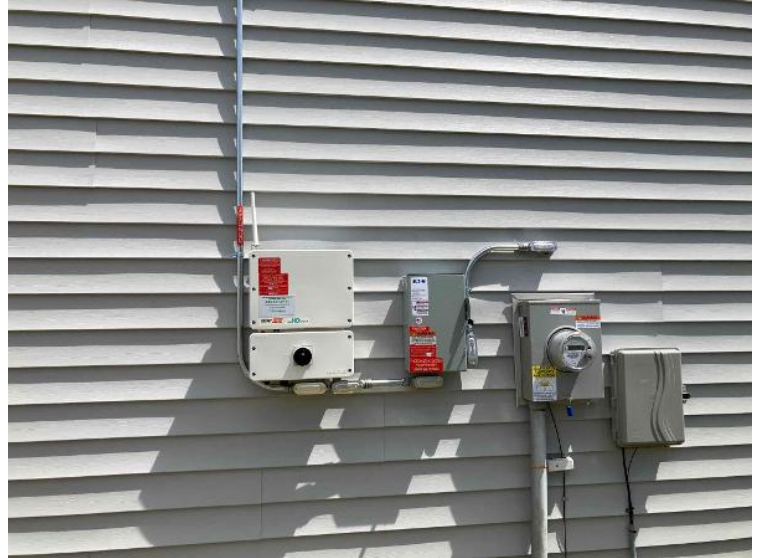
Project Completion Photos / Pullback Photos of All BOS Mounted in Completed State
