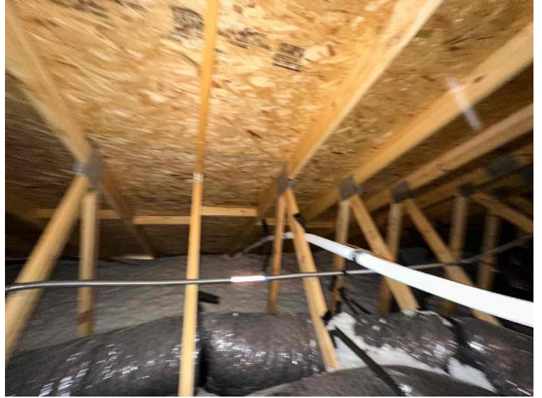
Rooftop Installation / Overall Conduit Run, Between Arrays, Attic Runs Included, Down To BOS
