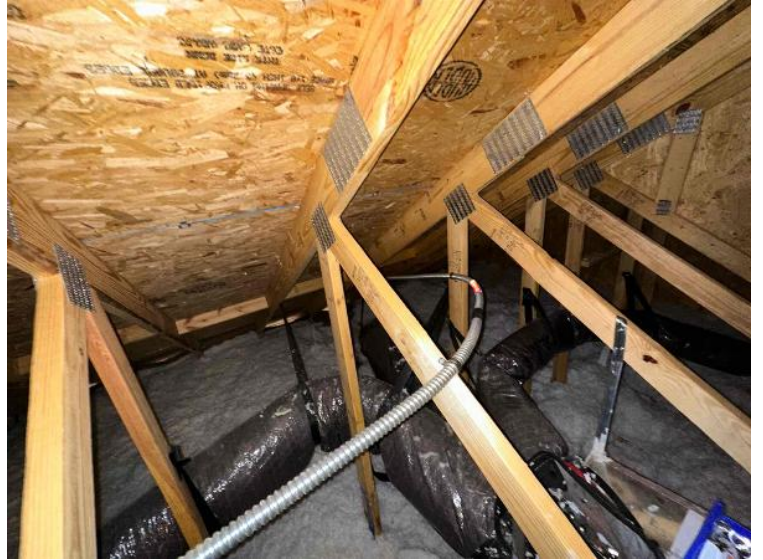
Rooftop Installation / Overall Conduit Run, Between Arrays, Attic Runs Included, Down To BOS
