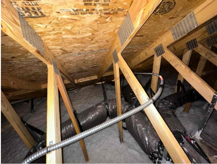
Rooftop Installation / Overall Conduit Run, Between Arrays, Attic Runs Included, Down To BOS
