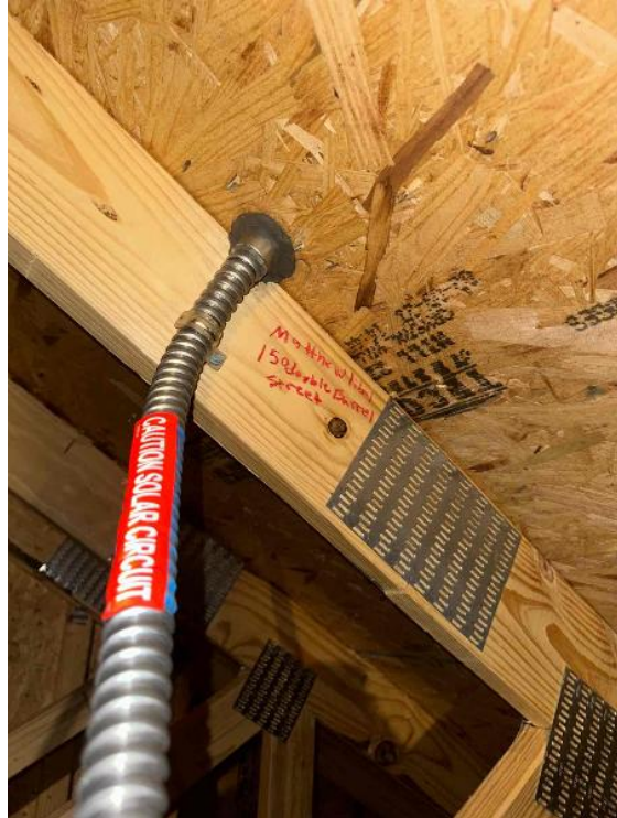
Rooftop Installation / Overall Conduit Run, Between Arrays, Attic Runs Included, Down To BOS
