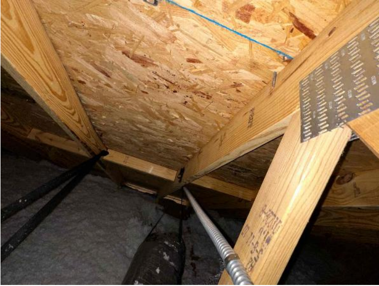
Rooftop Installation / Overall Conduit Run, Between Arrays, Attic Runs Included, Down To BOS
