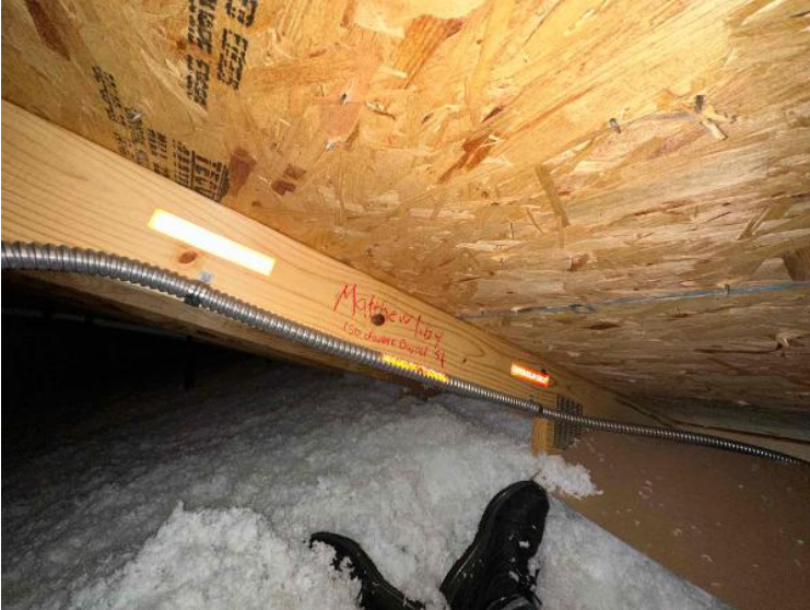
Rooftop Installation / Overall Conduit Run, Between Arrays, Attic Runs Included, Down To BOS
