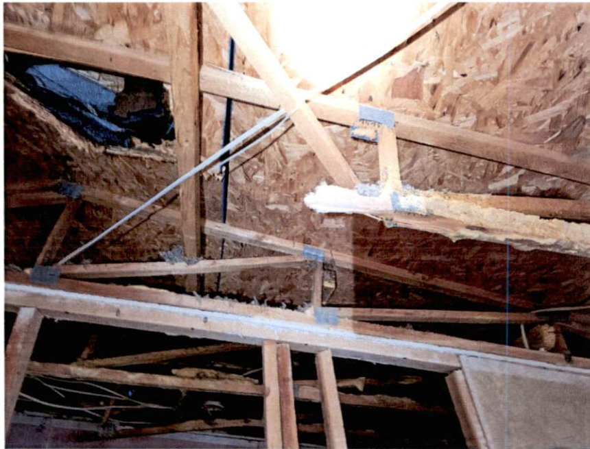
Picture 3 – Example of broken trusses in the back left bay of the home
