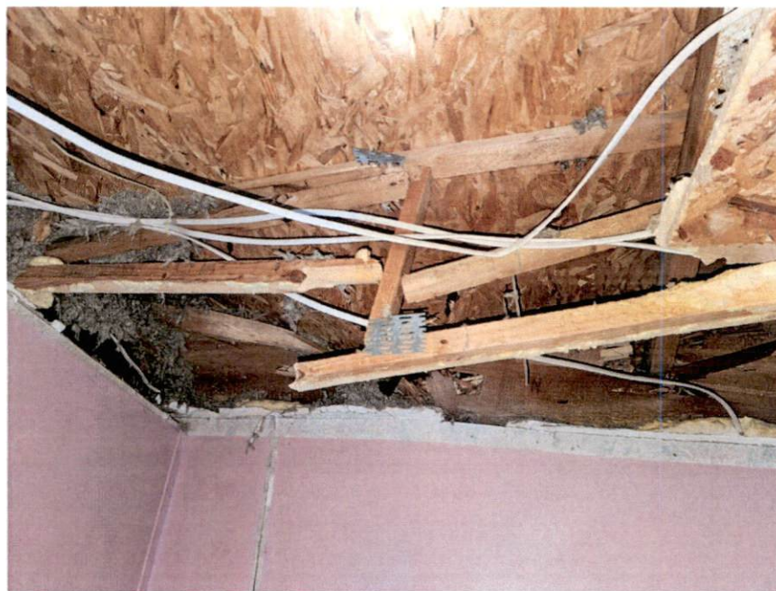
Picture 4 – Example of broken trusses in the back left bay of the home
