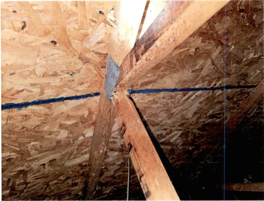
Picture 7 – Example of truss members not properly connected to the gusset plate
