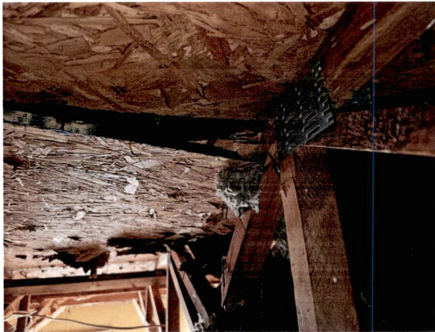
Picture 5 – Example of a damaged truss member in the front left bay of the home
