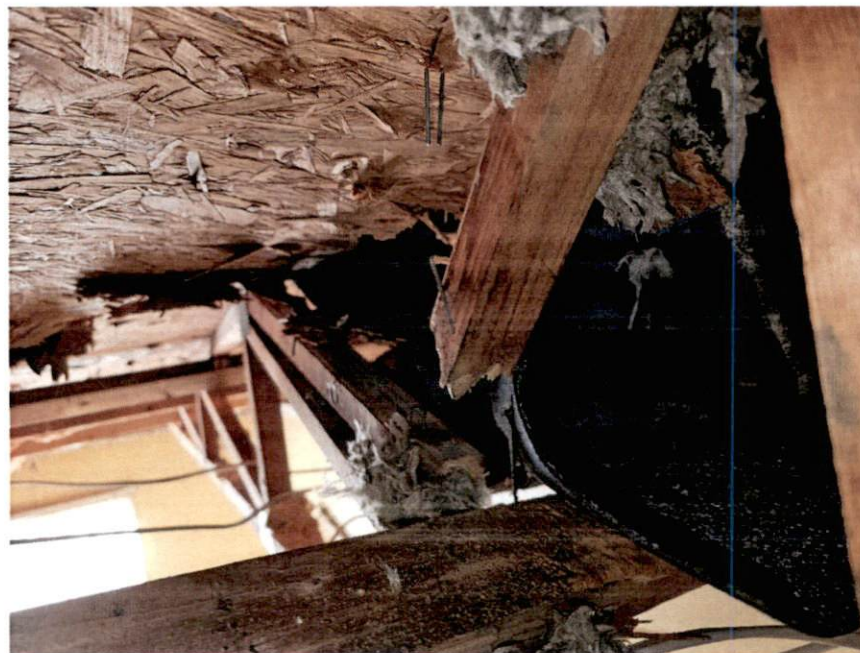
Picture 6 – Example of a damaged truss member in the front left bay of the home
