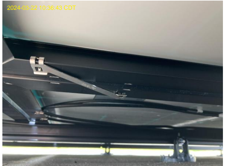
Modules / Grounding (All rows of modules, including bare copper, row-to-row ground clips, or bonding jumpers)
