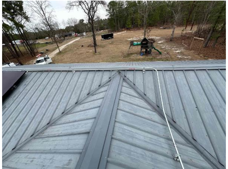
Rooftop Installation / Overall Conduit Run, Between Arrays, Attic Runs Included, Down To BOS
