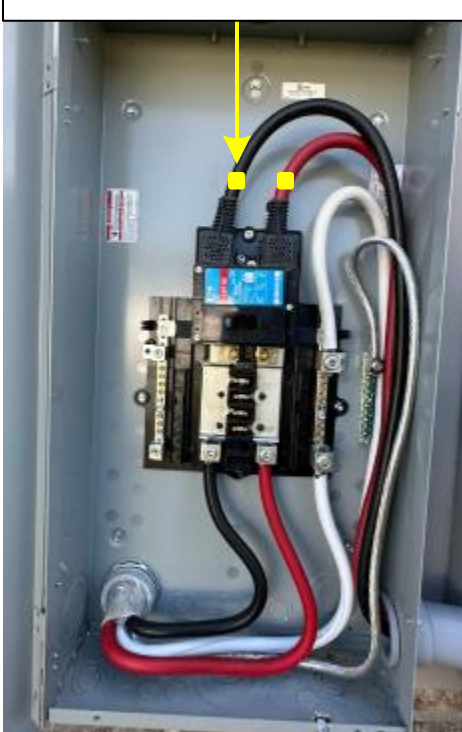
Line Side Tap inside the Main Load Panel
