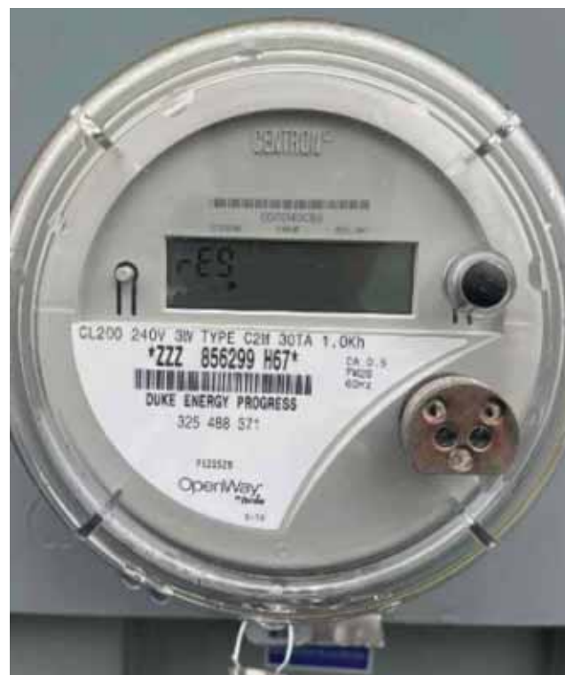
UTILITY COMPANY: Duke Energy NC
