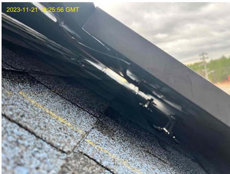
Roof/Array Information / Roof Array / Under Array (wire management)
