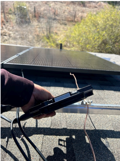
Detailed picture of micro inverter W/ reference point turned sideways with serial # visible
