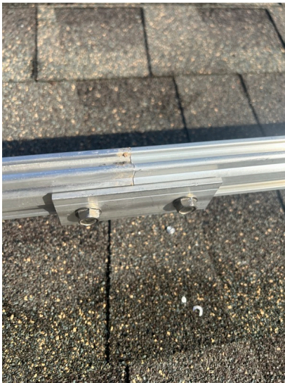
Detailed picture of rack splicing
