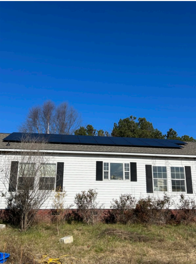
Pictures of completed arrays (all panels need to be captured)
