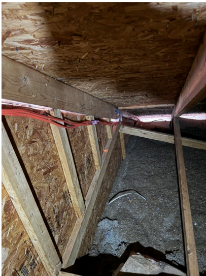
Detailed pictures of wires and cables used on roof
