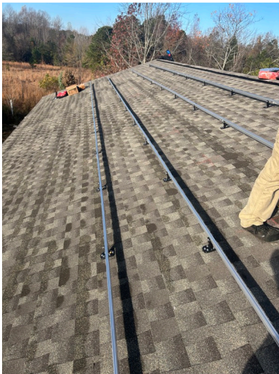
Detailed picture of complete racking installed
