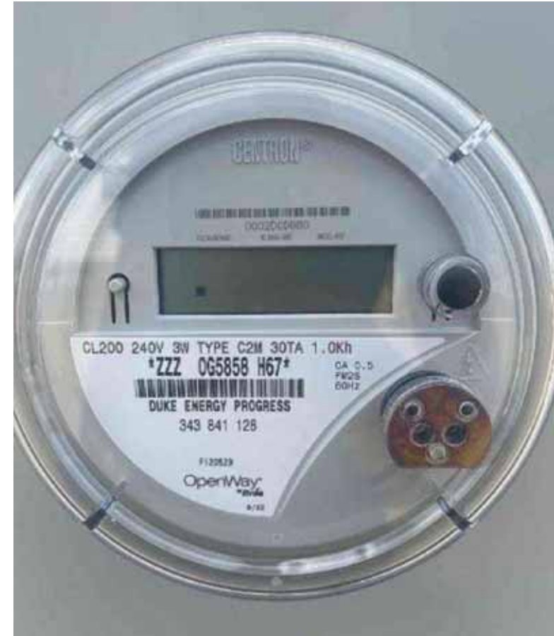
UTILITY COMPANY: Duke Energy NC
