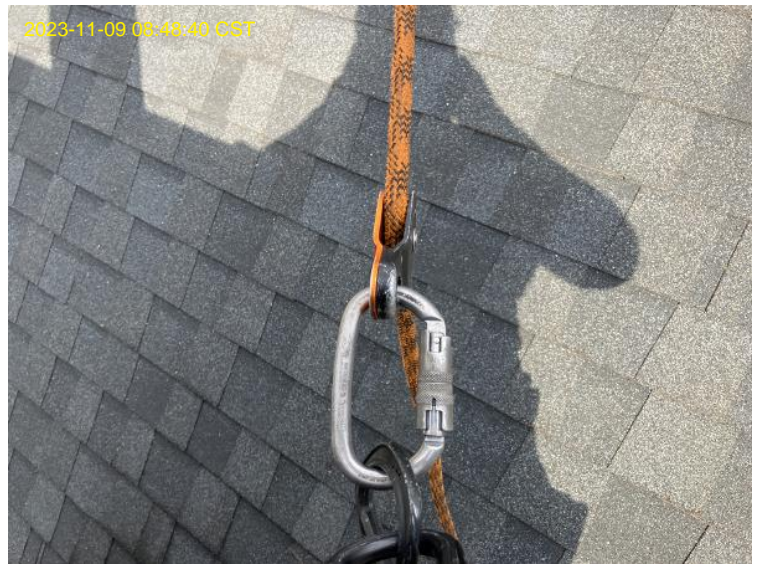
Safety / Fall Protection PPE (e.g, rope, caribiner)
