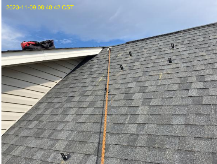
Safety / Fall Protection PPE (e.g, rope, caribiner)
