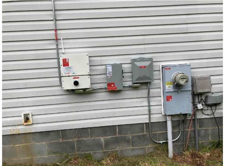
Electrical / Pullback Photo of Inverter Mounted
