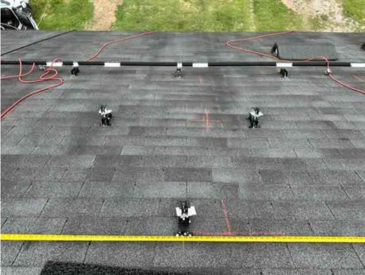
Module Installation / Ready for Modules (All rail-less parts required to land modules complete)
