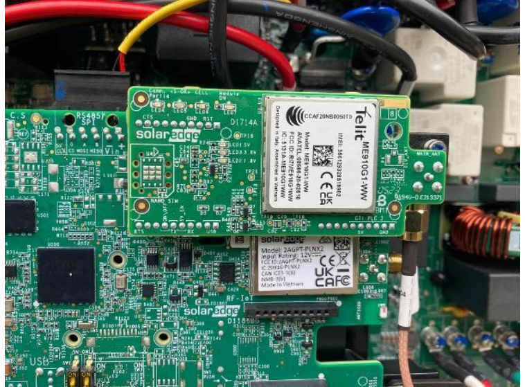
Electrical / Inverter Interior With Top/Bottom Cover off (cell kit installed + Wiring Completed)
