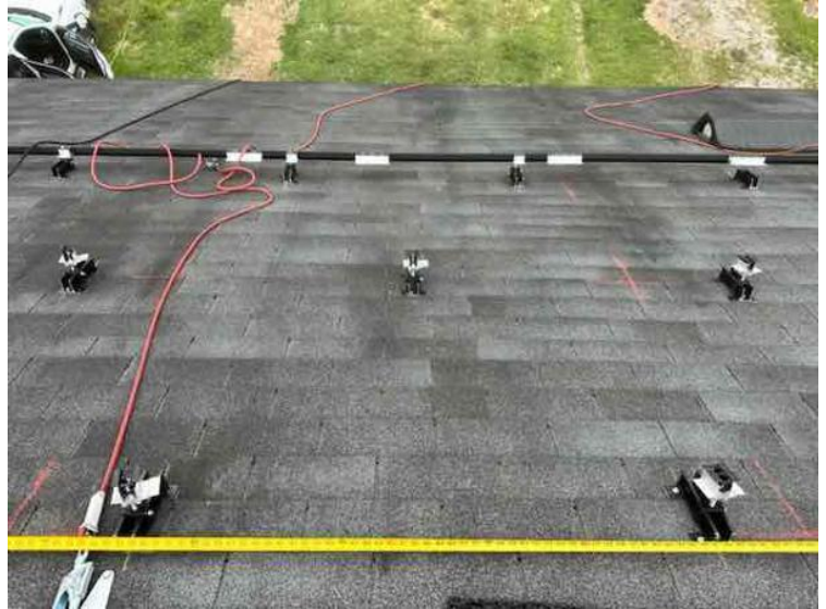
Module Installation / Ready for Modules (All rail-less parts required to land modules complete)
