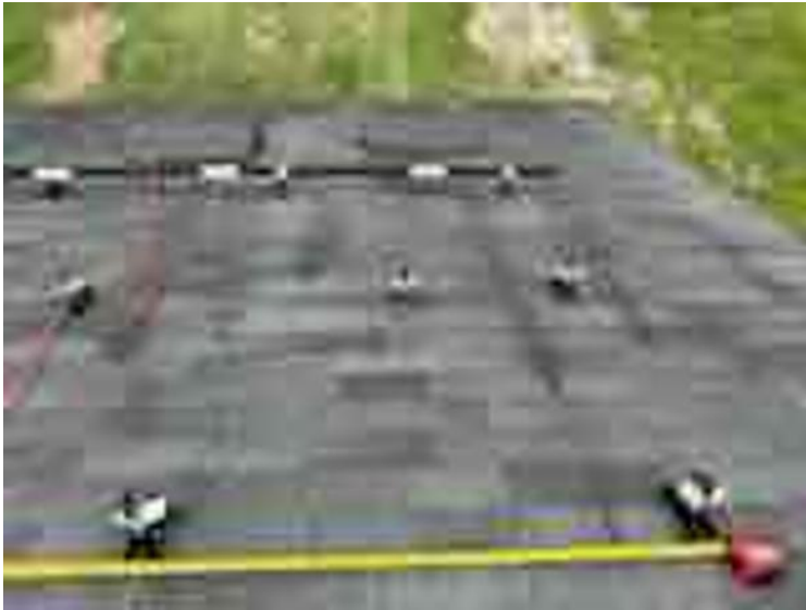
Module Installation / Ready for Modules (All rail-less parts required to land modules complete)
