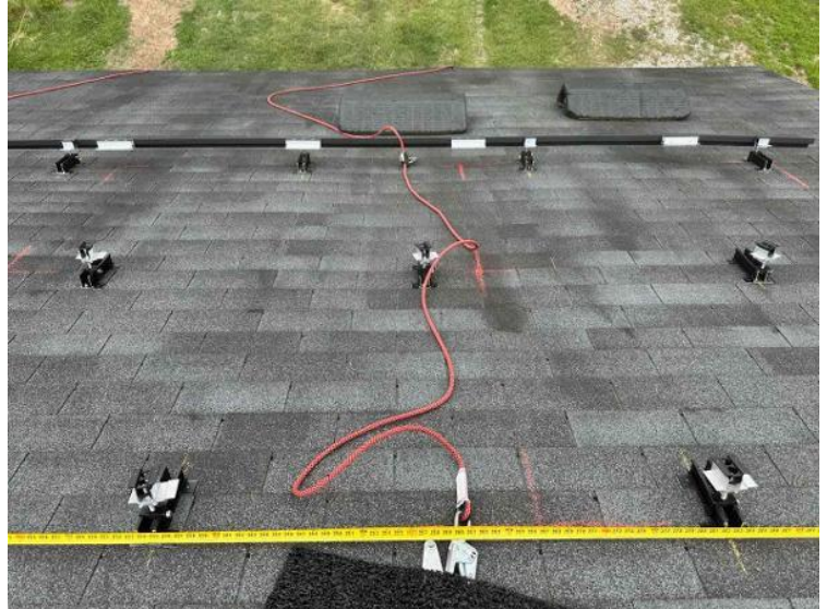
Module Installation / Ready for Modules (All rail-less parts required to land modules complete)
