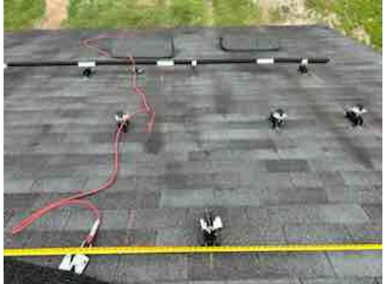
Module Installation / Ready for Modules (All rail-less parts required to land modules complete)
