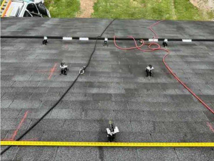
Module Installation / Ready for Modules (All rail-less parts required to land modules complete)
