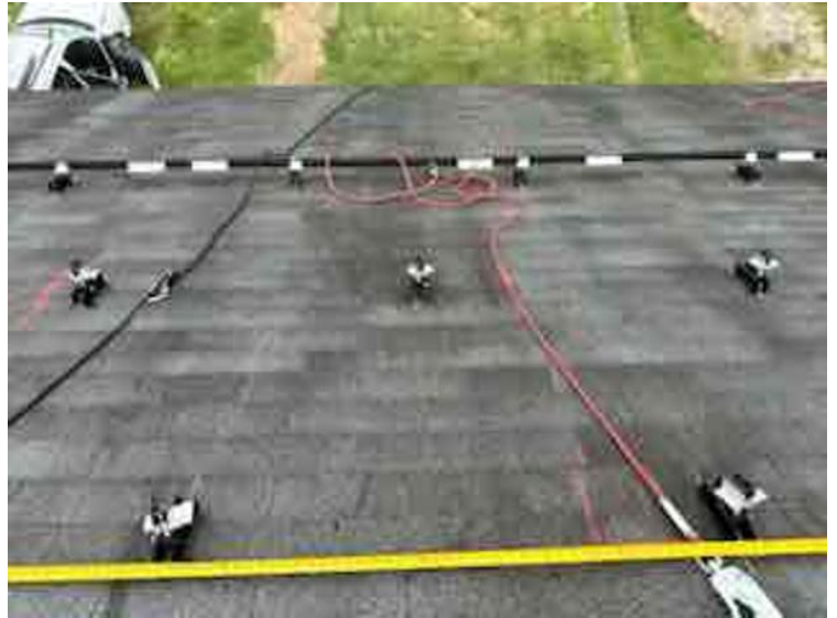
Module Installation / Ready for Modules (All rail-less parts required to land modules complete)
