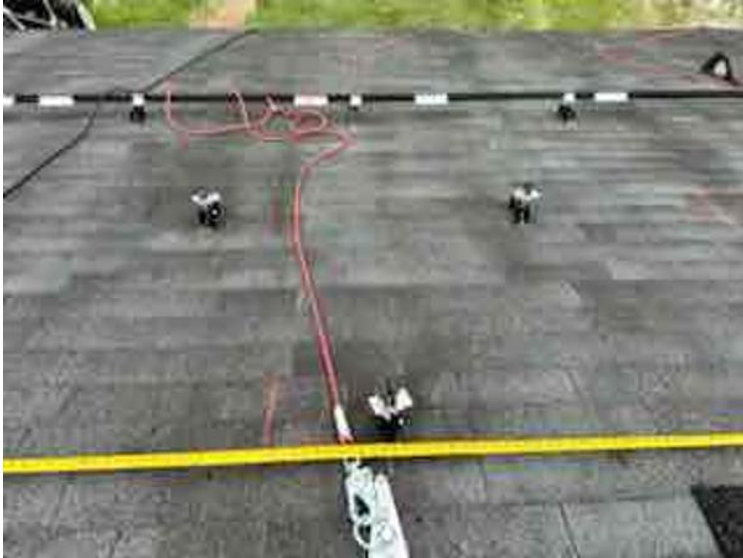
Module Installation / Ready for Modules (All rail-less parts required to land modules complete)
