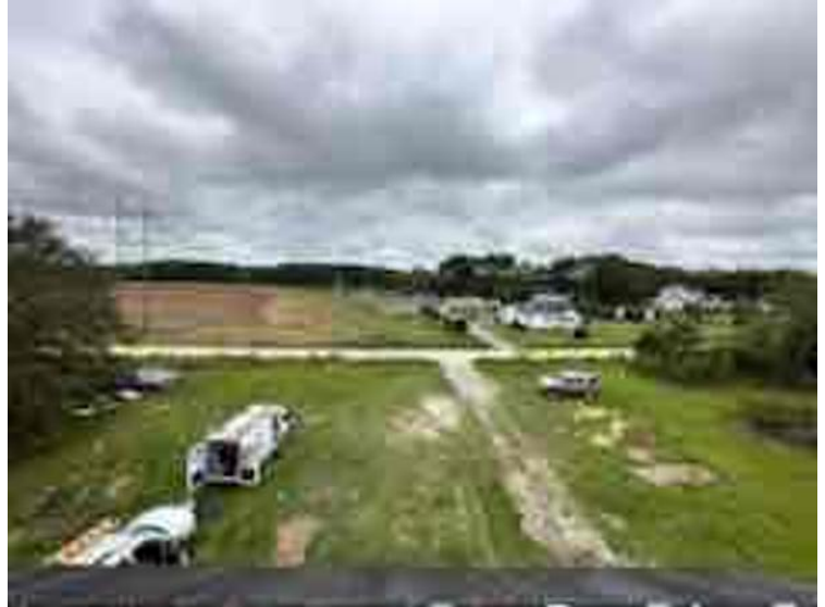
Module Installation / Ready for Modules (All rail-less parts required to land modules complete)
