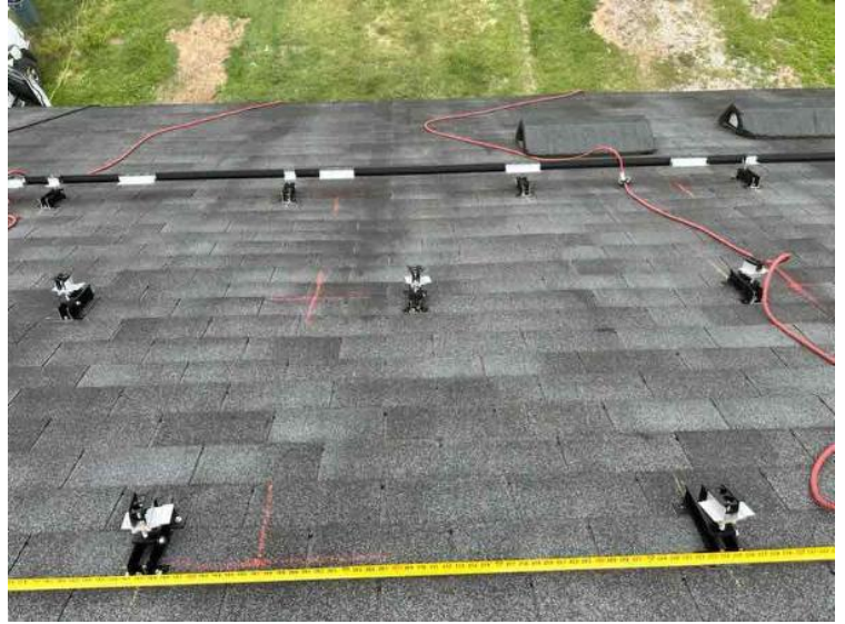
Module Installation / Ready for Modules (All rail-less parts required to land modules complete)
