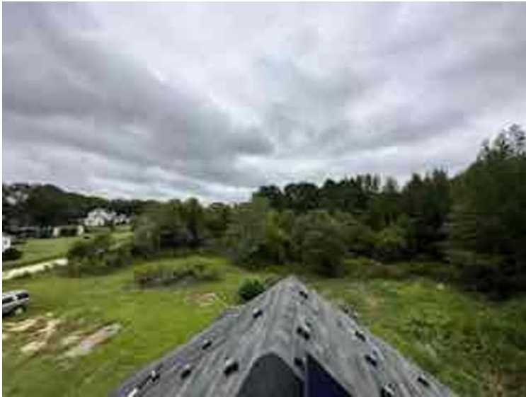
Module Installation / Ready for Modules (All rail-less parts required to land modules complete)
