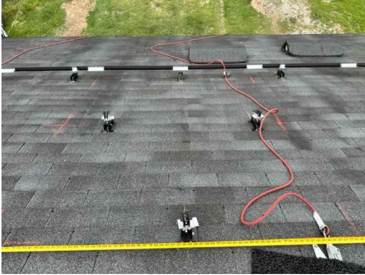
Module Installation / Ready for Modules (All rail-less parts required to land modules complete)
