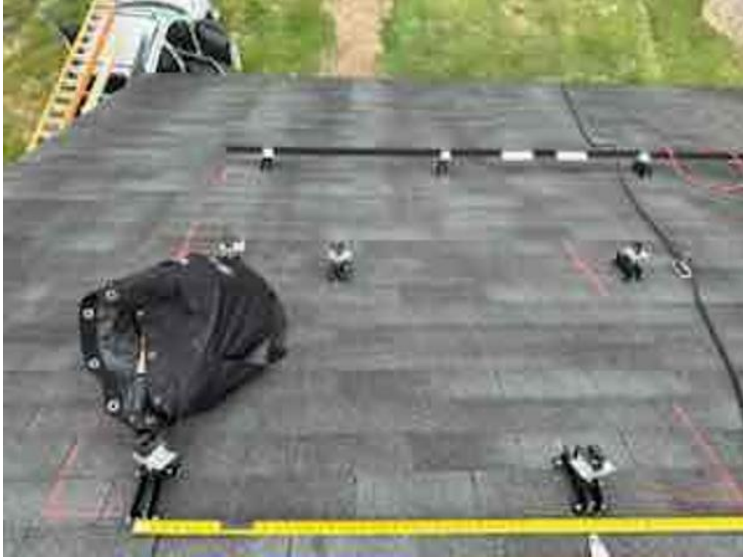
Module Installation / Ready for Modules (All rail-less parts required to land modules complete)
