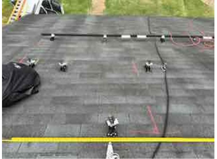
Module Installation / Ready for Modules (All rail-less parts required to land modules complete)
