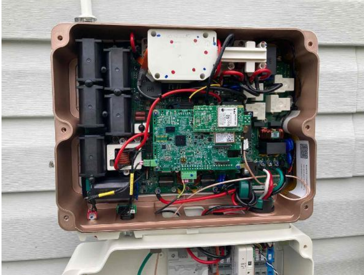
Electrical / Inverter Interior With Top/Bottom Cover off (cell kit installed + Wiring Completed)
