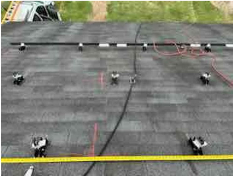
Module Installation / Ready for Modules (All rail-less parts required to land modules complete)
