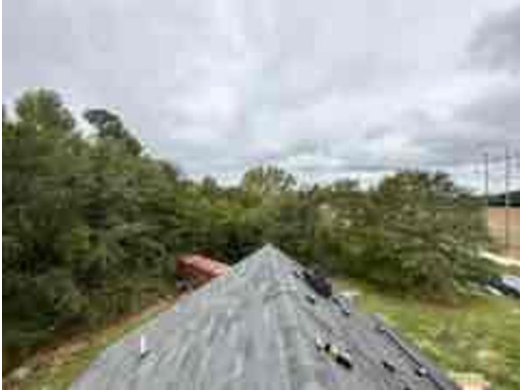
Module Installation / Ready for Modules (All rail-less parts required to land modules complete)
