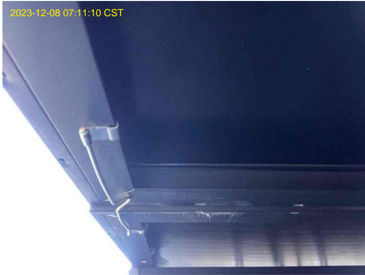
Modules / Grounding (All rows of modules, including bare copper, row-to-row ground clips, or bonding jumpers)
