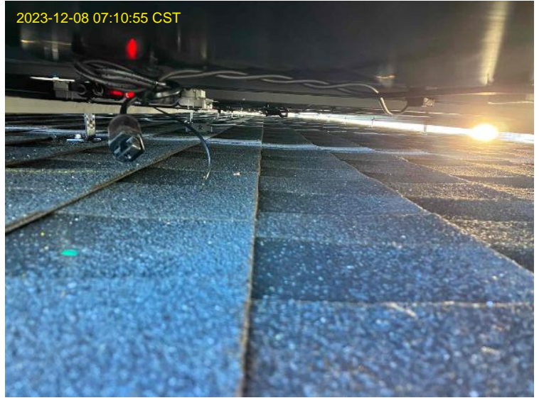
Modules / Wire Management - Under Array (Can be taken from GROUND)
