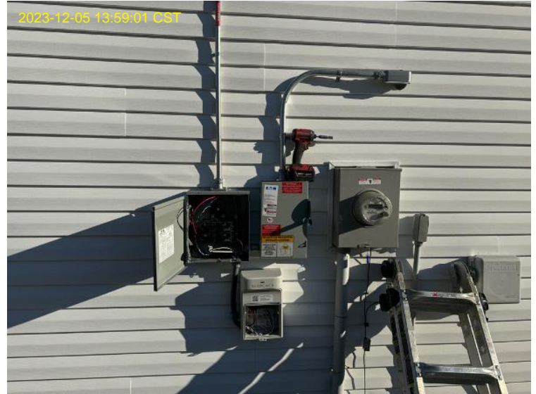
Interior of Enclosures / Wide Shot: EQ Wall w/o Deadfronts - Indoor & Outdoor
