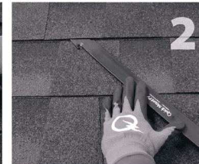
2 Carefully lift composition roof shingle with roofing bar, just above placement of mount. Remove nails as required and backfill holes with approved sealant. See "Proper Flashing Placement" on next page.
