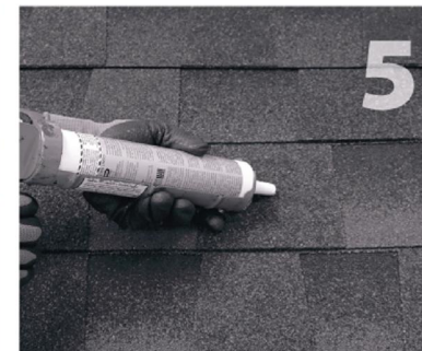
5 Clean off any sawdust, and fill hole with sealant compatible with roofing materials.
